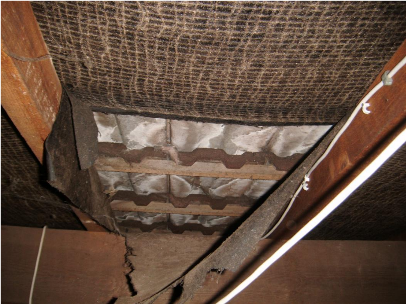
Some peeled bitumen felt in loft
