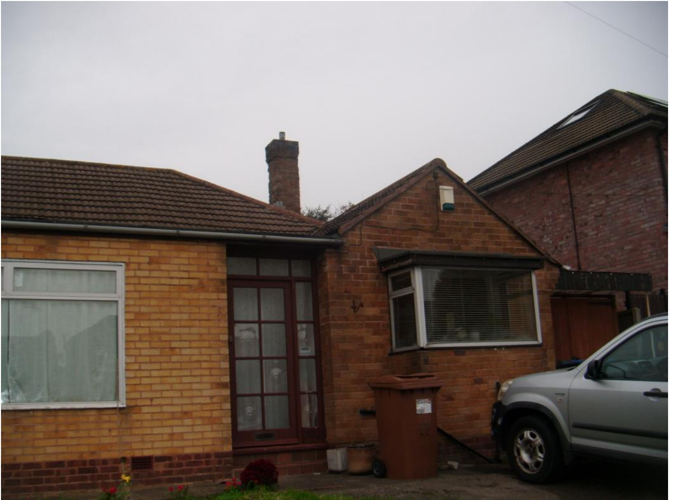
Front intact tiles
