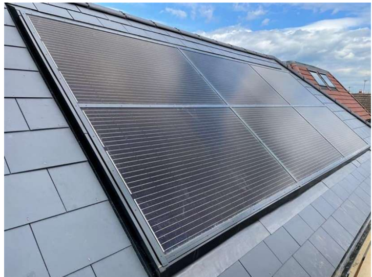
Photovoltaic Solar Panels
