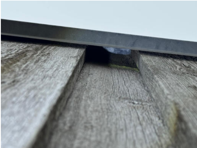
Photo 3: Open soffit voids
