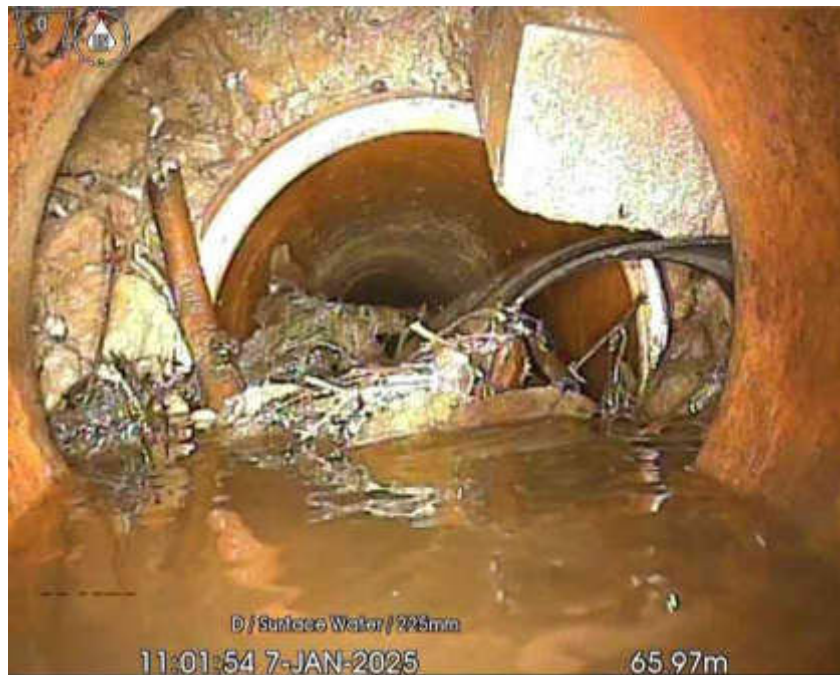
SW03X_D_07012025_1048_003.jpg, 00:07:06, 65.97 m Hole in drain or sewer from 7 o'clock to 5 o'clock
