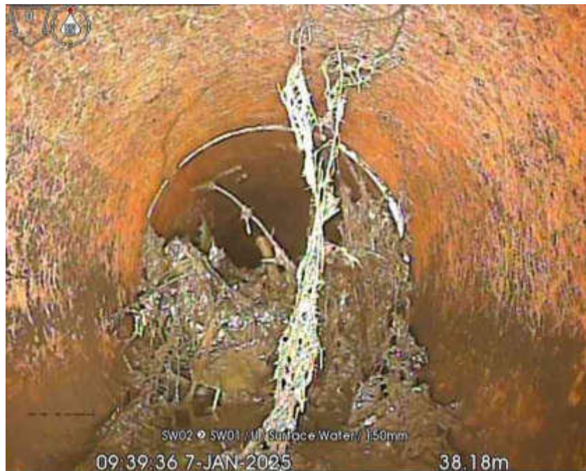
SW01X_U_07012025_0924_001.jpg, 00:05:12, 38.18 m Roots, mass, 50% cross-sectional area loss
