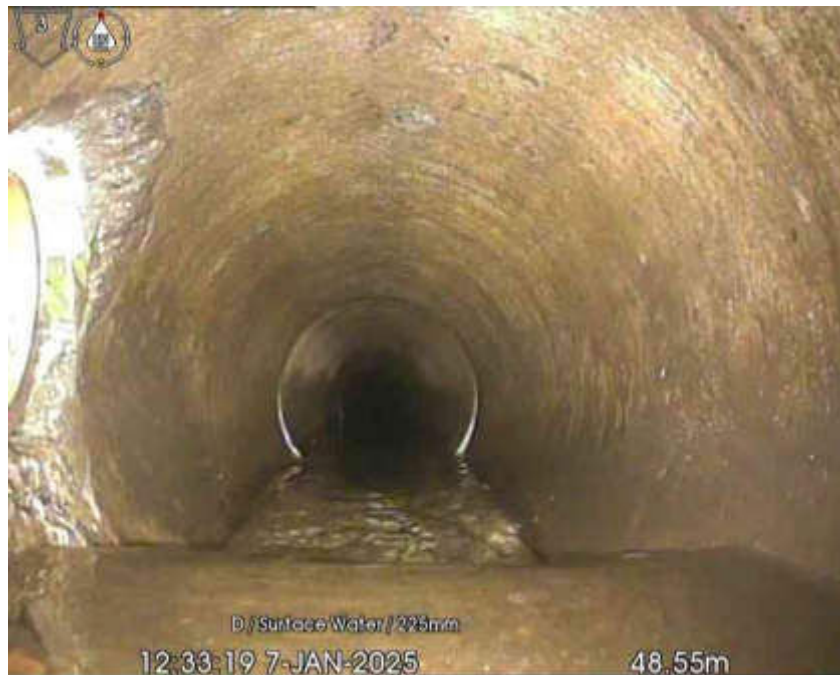
SW06X_D_07012025_1225_007.jpg, 00:06:02, 48.55 m Settled deposits, coarse, 10% cross-sectional area loss, finish
