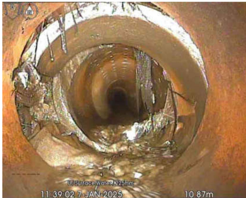
SW03X_U_07012025_1134_005.jpg, 00:01:32, 10.87 m Joint displaced, large
