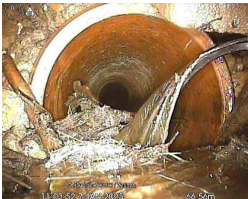
SW03X_D_07012025_1048_004.jpg, 00:08:48, 66.56 m Settled deposits, coarse, 30% cross-sectional area loss
