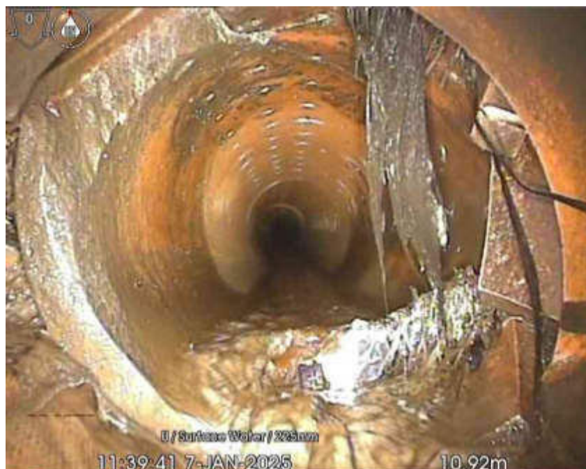
SW03X_U_07012025_1134_006.jpg, 00:01:32, 10.87 m Joint displaced, large
