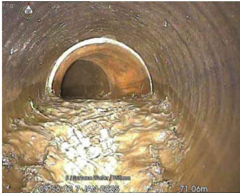
0703X_U_07012025_0944_002.jpg, 00:10:04, 71.06 m Roots, mass, 40% cross-sectional area loss
