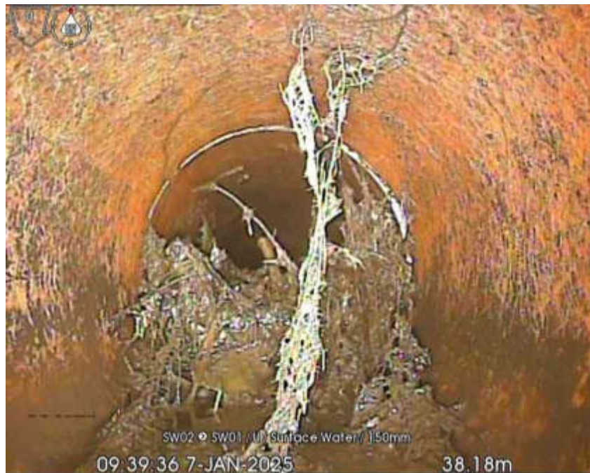
SW01X_U_07012025_0924_001.jpg, 00:05:12, 38.18 m Roots, mass, 50% cross-sectional area loss
