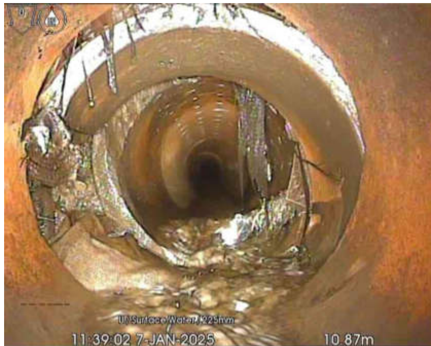
SW03X_U_07012025_1134_005.jpg, 00:01:32, 10.87 m Joint displaced, large
