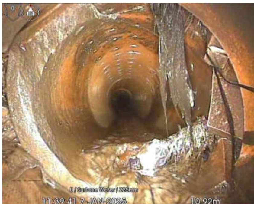
SW03X_U_07012025_1134_006.jpg, 00:01:32, 10.87 m Joint displaced, large
