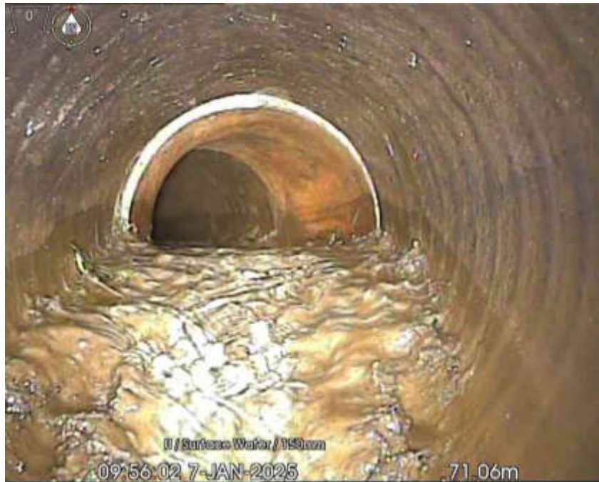
0703X_U_07012025_0944_002.jpg, 00:10:04, 71.06 m Roots, mass, 40% cross-sectional area loss
