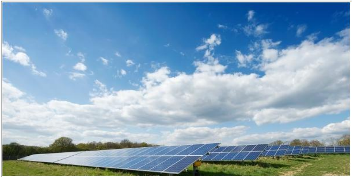
Figure 4.1: A Typical Operational Solar Farm
