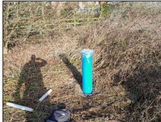
5. Instruments deployed on site within raised headworks.
