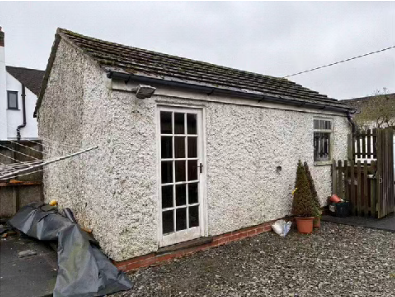
The side large single storey garage facing the house. The textured render is not weathering well.
