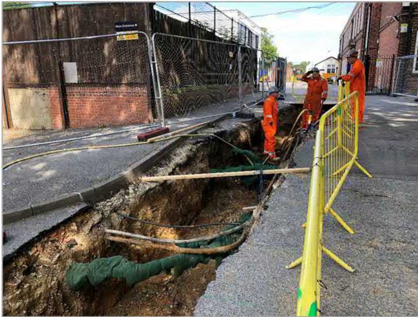
Figure 5 – Retained roots in service trench.
