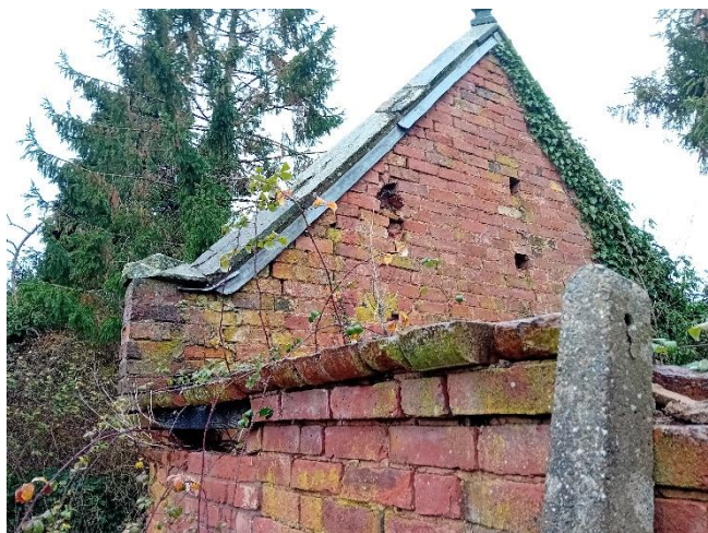
Photo 7: Gaps in the mortar on the east elevation of the west gable wall of building B1.
