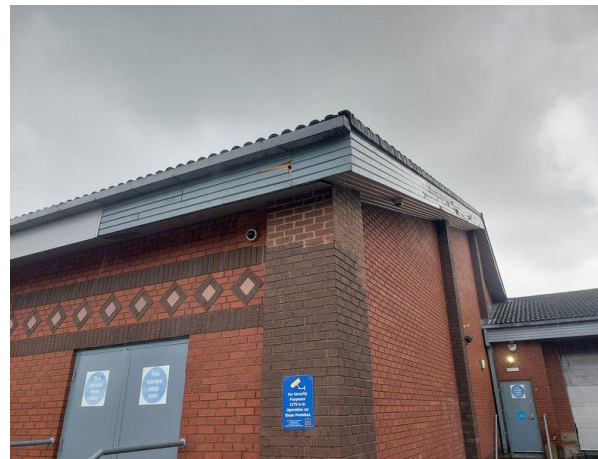
Plate 9.10: Damaged soffit on north-east corner of the building
