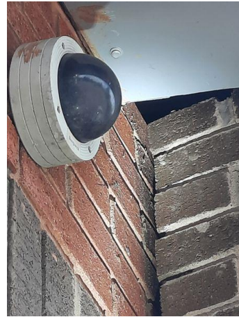
Plate 9.8: Example of a gap between wall and soffit
