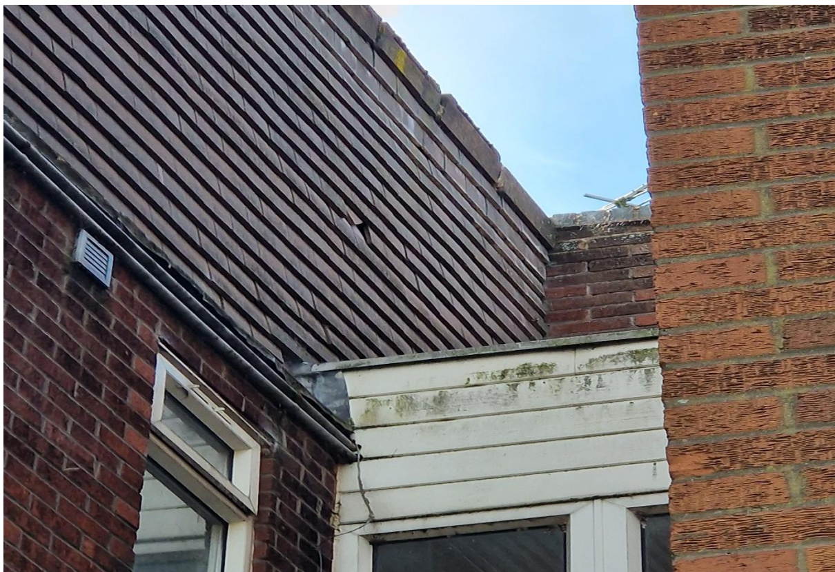
Plate12: Image showing the missing edge tile on B1 .
