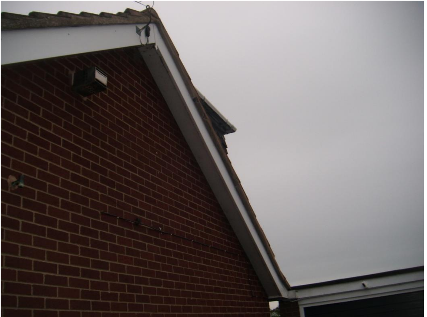
Gable end intact
