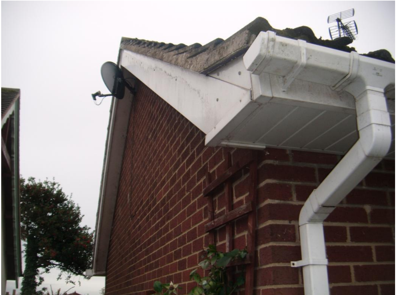
Gable end intact
