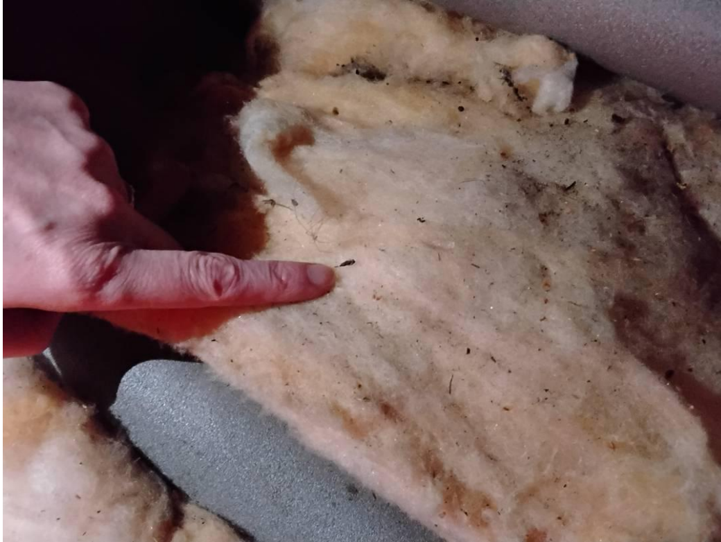
Photo 15. Bat droppings located within the void of B1.
