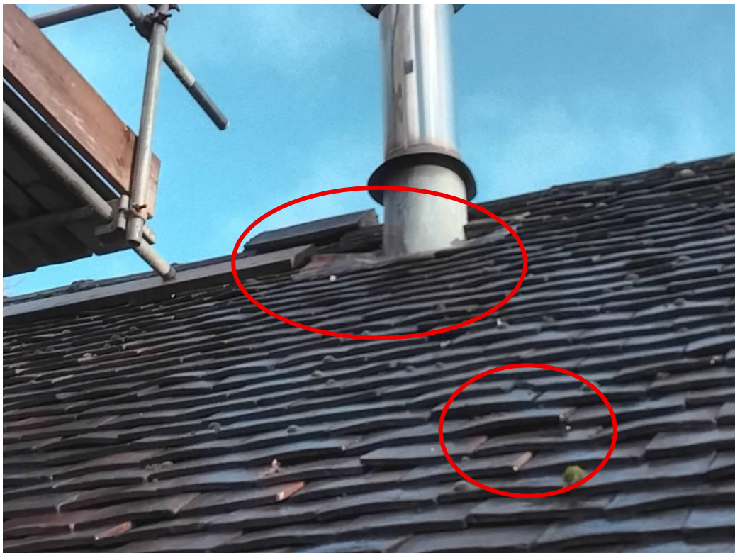
Photo 12. Various access points at the tile ridge, lead flashing and raised tiles
