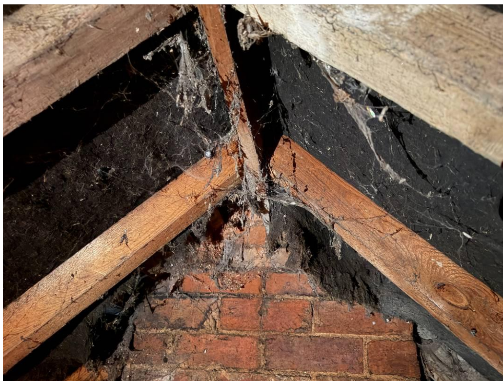
Photo 14. Heavily cobwebbed area directly adjacent to the chimney.
