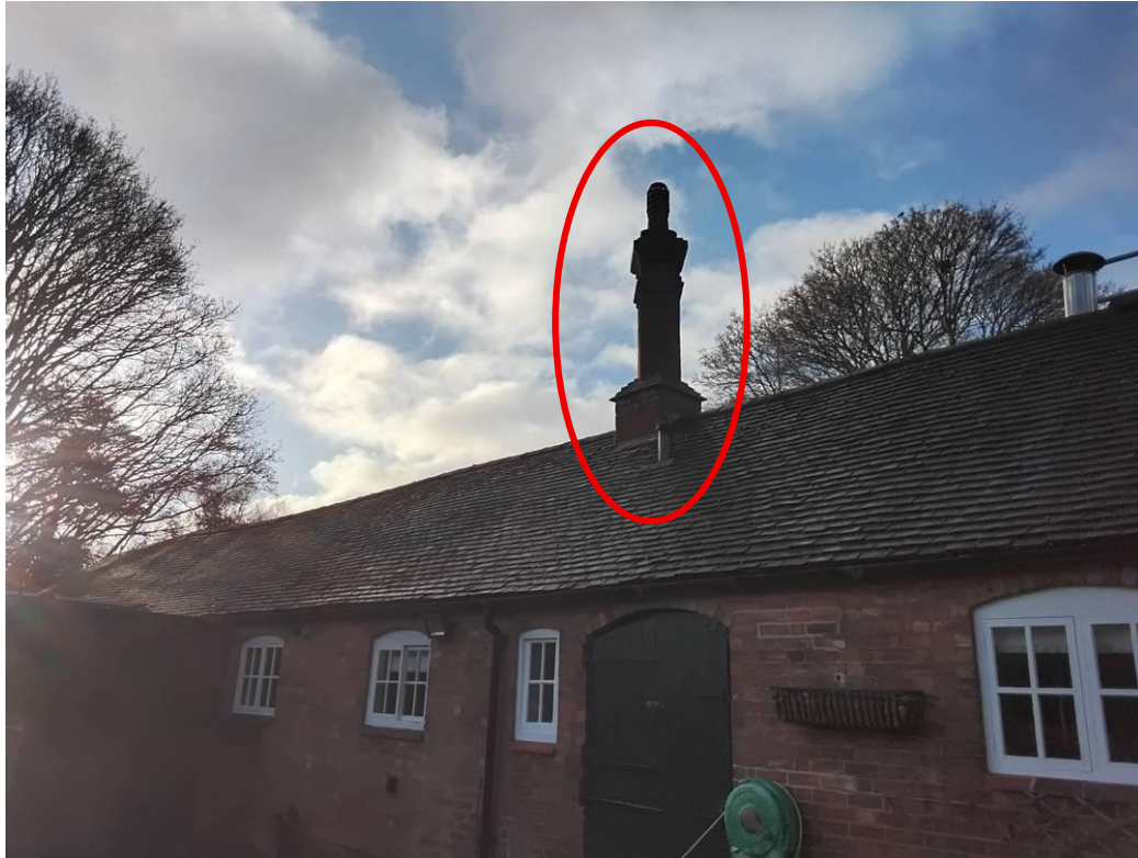
Photo 11. B1, with the chimney affected by the works circled in red.
