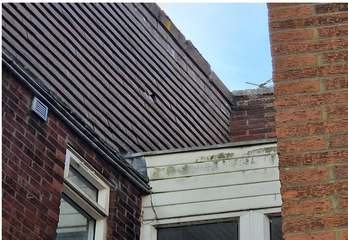
Plate12: Image showing the missing edge tile on B1 .
