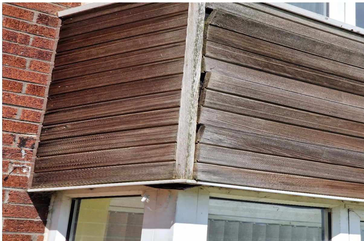
Plate 15: Image showing loose wood panels on B3 .
