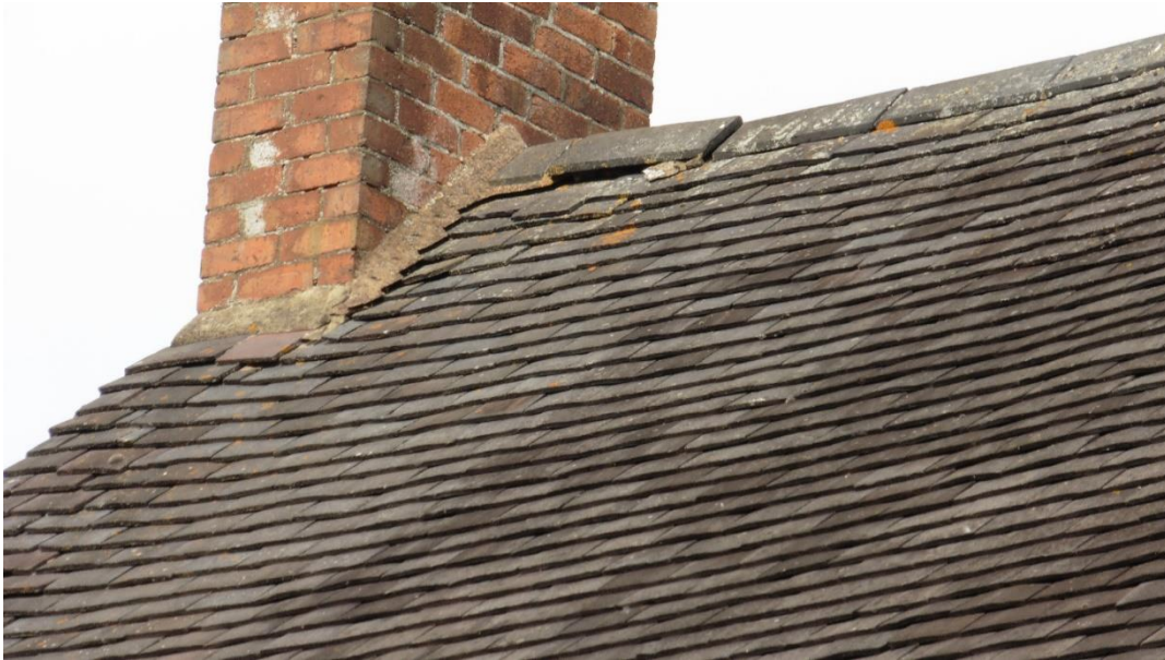
Photograph 8: example of potential bat roosting feature under ridge tiles on the main traditional house.
