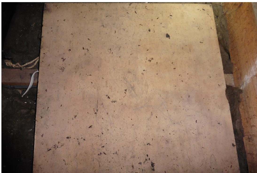
Photograph 5 - Pipistrelle droppings below the ridgeboard in the north-east extension
