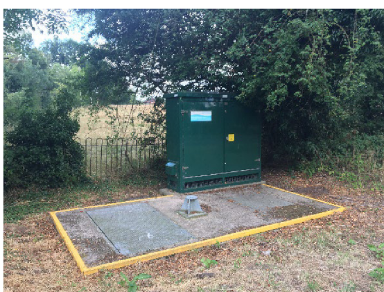
Photo 11: Severn Trent Sewage Pumping Station north of Field 2
