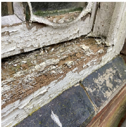
Rotten windows to cottage to be replaced with timber sash to match original.
