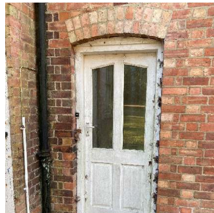
Modern door to Cottage to be replaced with new timber door.
