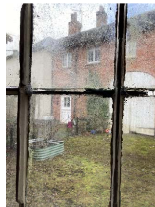
Figure 30. Cottage, missing and rotten glazing bars (Savills: 2024)
