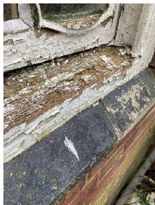
Figure 29. Cottage, typical rotten sill (Savills: 2024)
