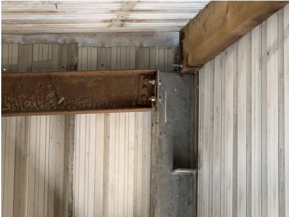
Photograph 5 – Distortion of the rafter/stanchion connection at eaves level
