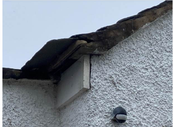
Gaps along roof edge north side of house
