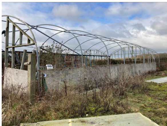
Derelict polytunnel frame.
