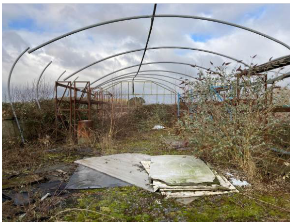
Derelict polytunnel frame
