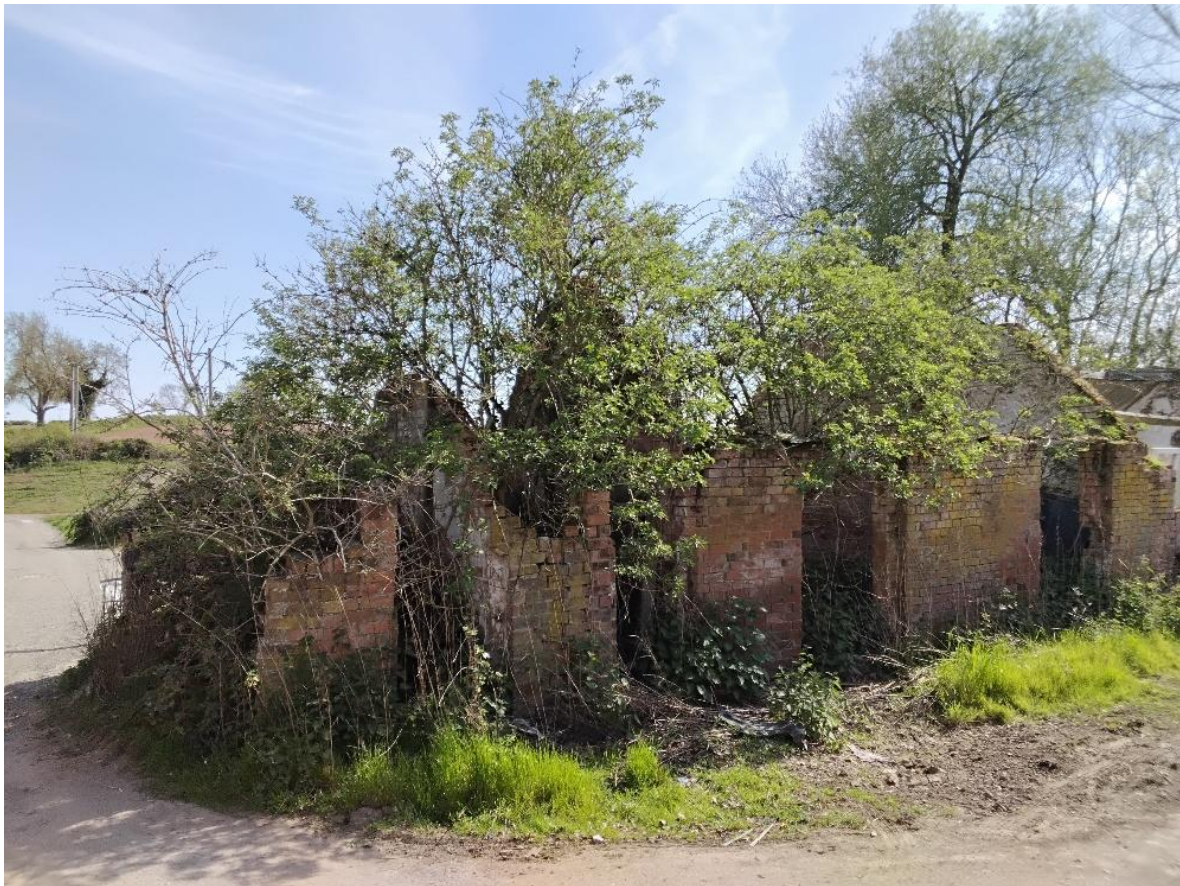
Photo 1. Former stable block in dilapidated condition with scrub colonising the eastern sections
