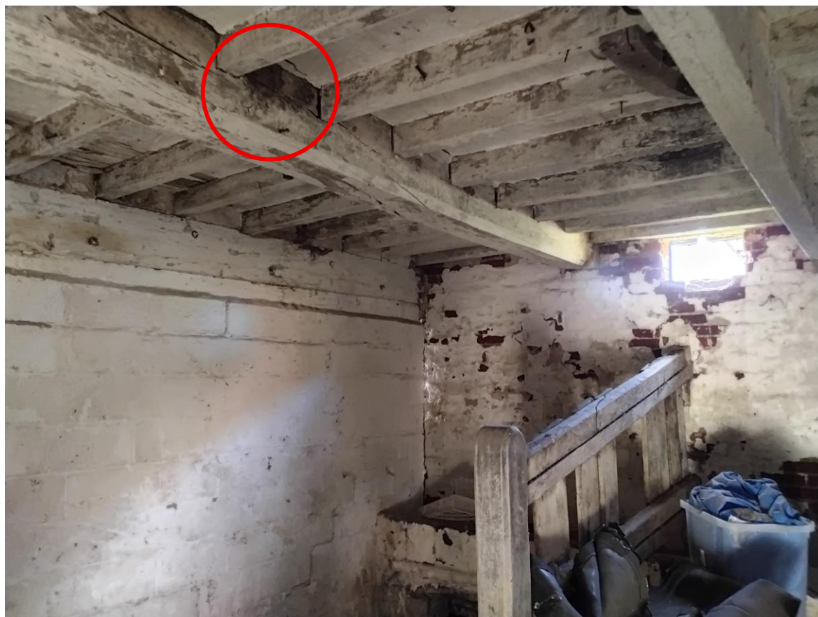
Photo 4: Western ground floor room, with birds' nest on the joist (circled).
