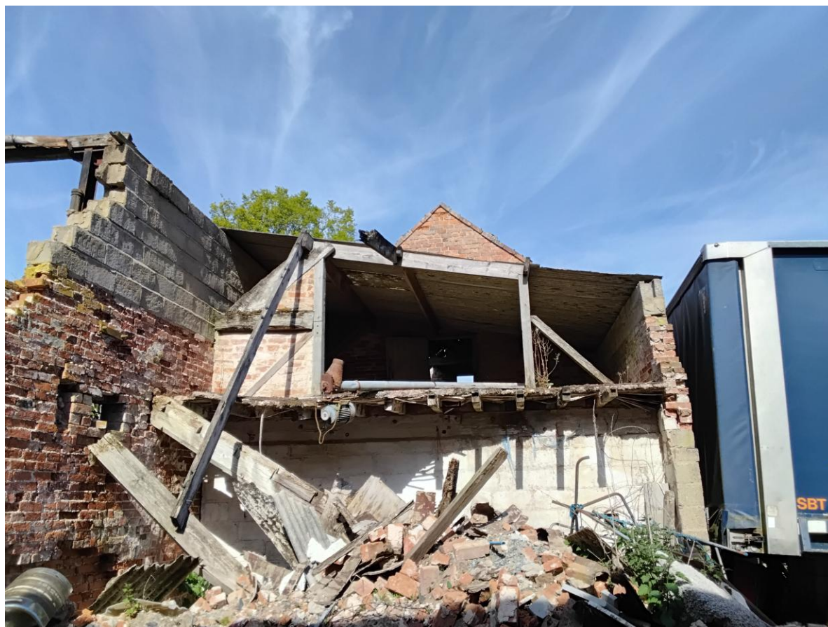
Photo 2: Partially collapsed western end of the building.
