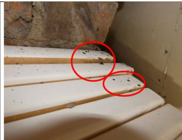
Photograph 27. Bat droppings within the western section of enclosed roof void under the chimney
