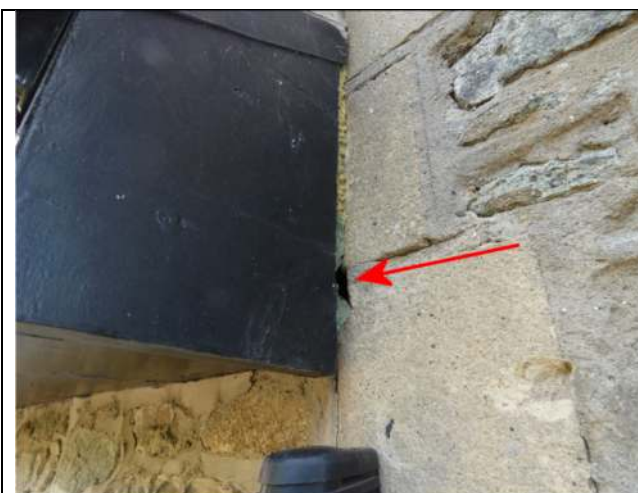
Photograph 17. Gap between the wall and the soffit to the east of the westernmost north-facing dormer window
