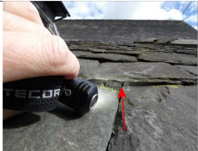
Photograph 10. Further example of an opening under slates on the roof of the single-storey extension of the south-west corner of the house
