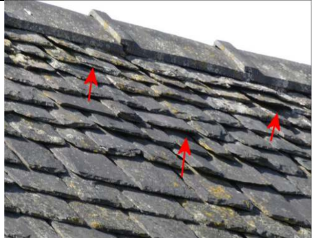
Photograph 8. Further example of openings under slates on the main roof of the house
