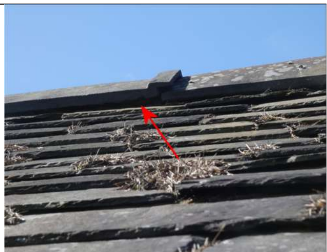
Photograph 36. Further example of an opening under a ridge tile on the roof of the outbuilding
