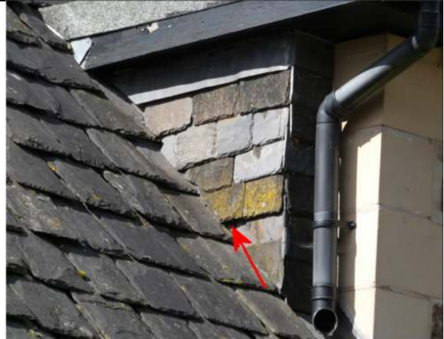
Photograph 14. Example of openings under hanging slates on the westernmost north-facing dormer window
