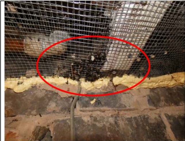
Photograph 19. Large accumulation of bat droppings in the boiler room to the east of the westernmost north facing dormer window
