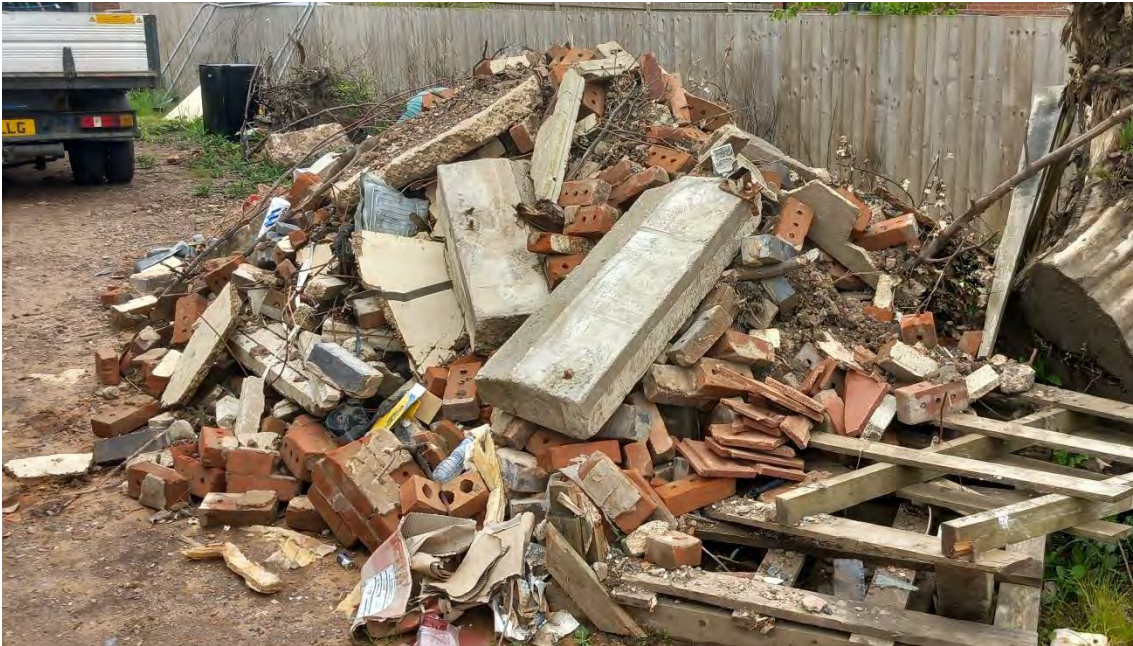
Rubble pile on western site boundary
