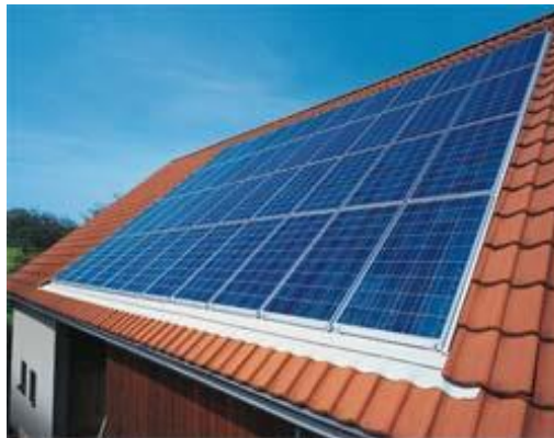
Figure 5.4 – A typical polycrystalline panel.
