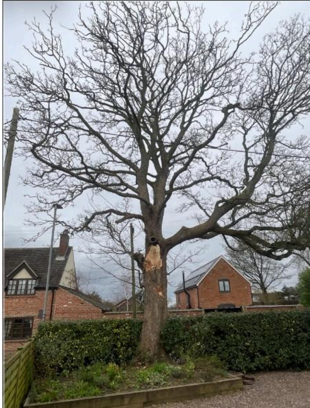
Photo 3 showing location of large limb failure (taken in December 2024)
