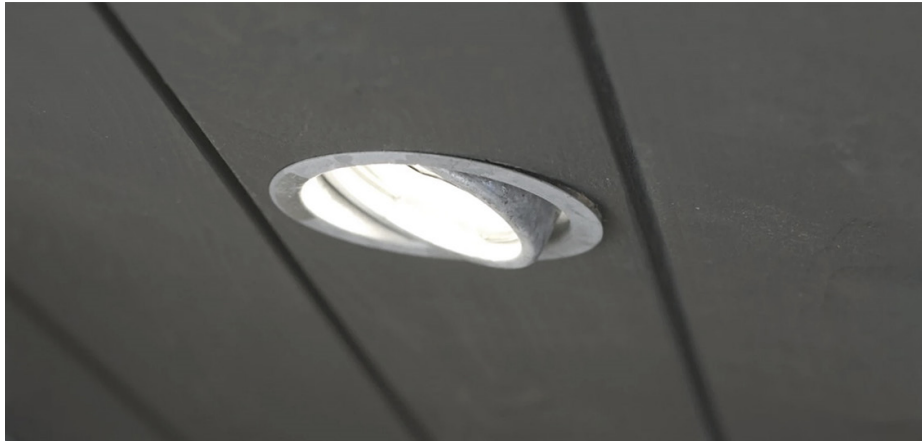
Figure 4 - Outdoor recessed LED downlights
