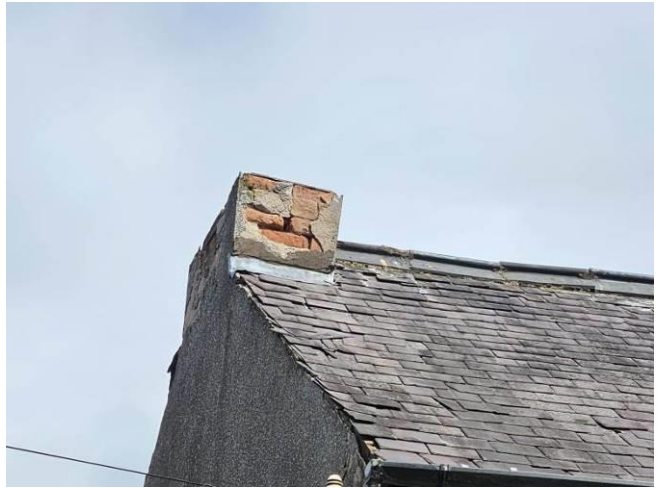
Damage to chimney and north eaves of western building
