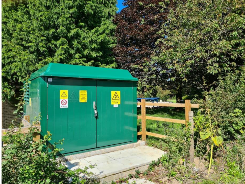
(Figure 2: Image of an example of the type of substation proposed. Please see accompanying plans for exact details of measurement and material use)
