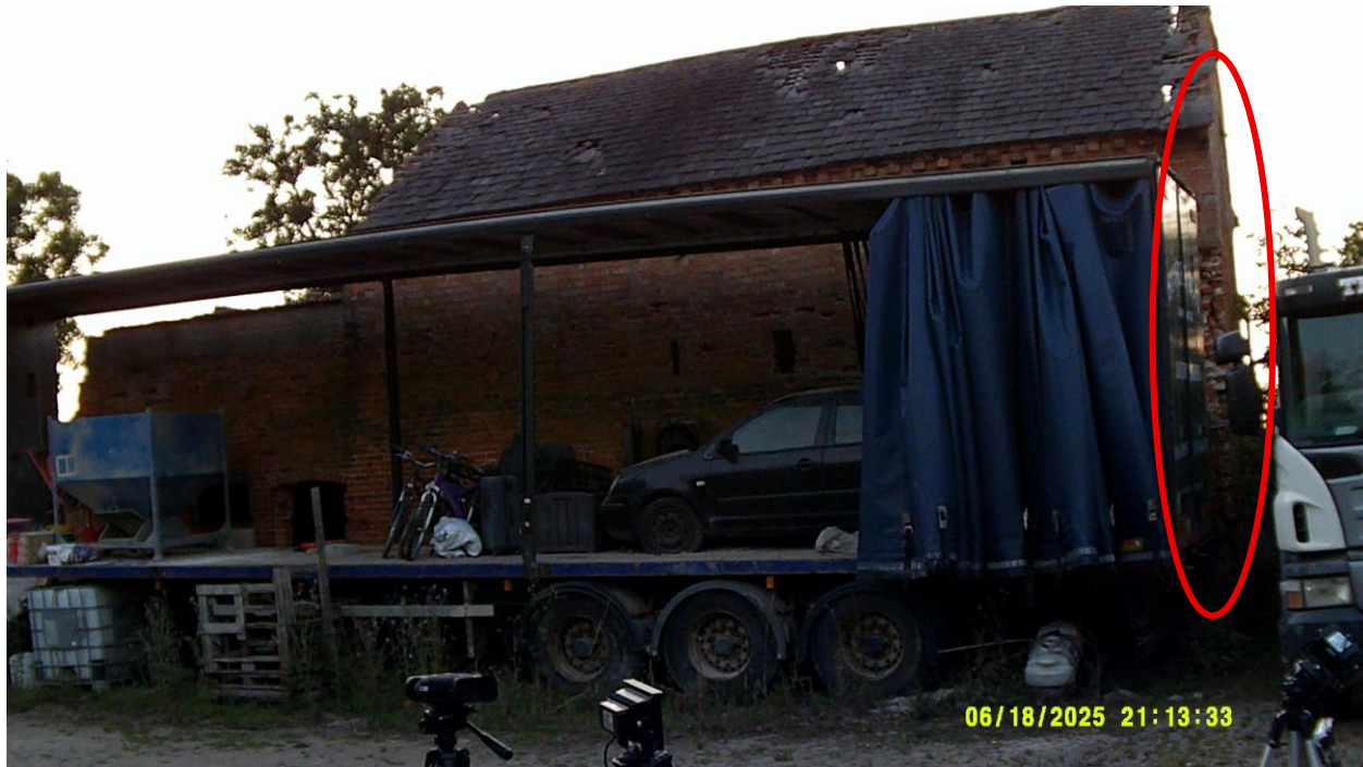
Photo 1: Southern elevation of the building, with fissure at the eastern end visible at the right end of the trailer (circled), and light visible through the roof gaps.
