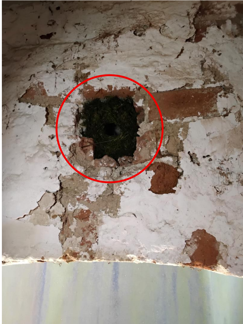
Photo 5: Nest in brickwork above door on the southern elevation
