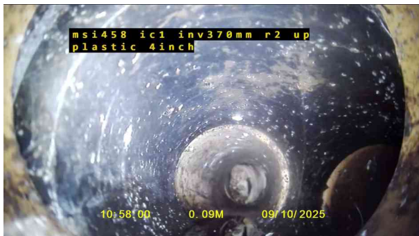
3, 00:00:08, 0.09 m Joint displaced, medium
