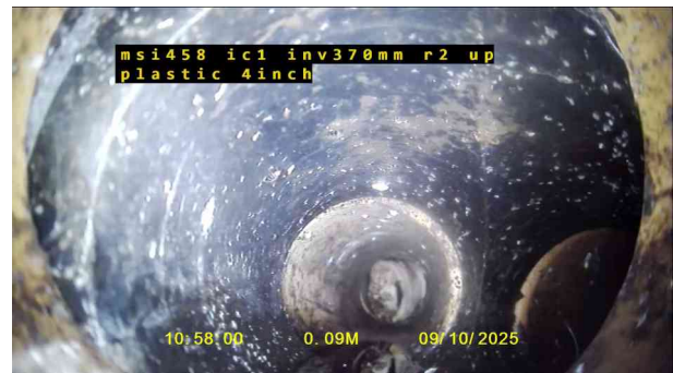
4, 00:00:08, 0.09 m Joint displaced, medium
