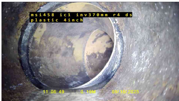
7, 00:00:11, 0.19 m Pipe material changes to polyvinyl chloride at this point
