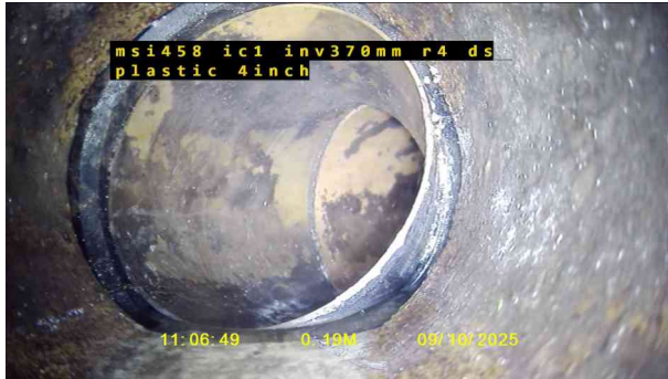
5, 00:00:11, 0.19 m Joint displaced, large
