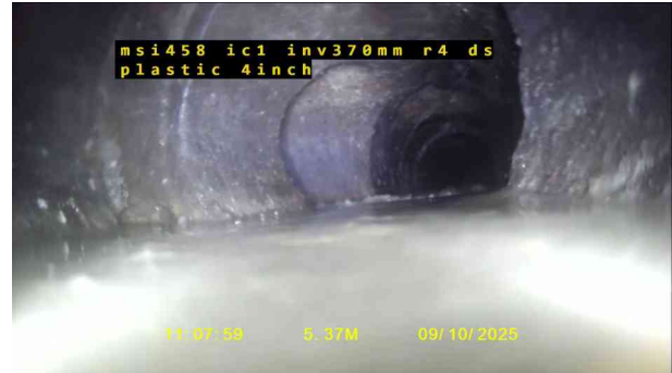
2, 00:01:21, 0.00 m Junction at 9 o'clock, 100mm dia
