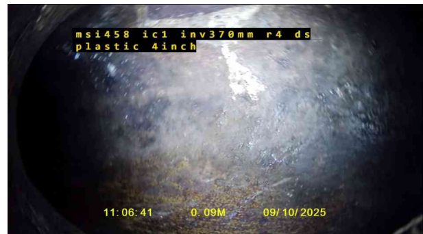
4, 00:00:04, 0.09 m Pipe material changes to vitrified clay at this point
