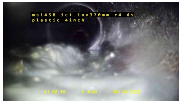
14, 00:01:38, 6.72 m Joint displaced, medium
