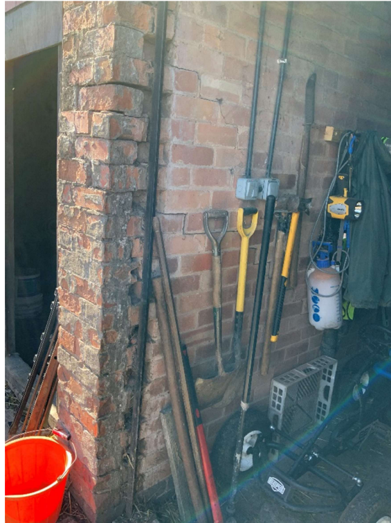
Picture 23 – Closer view of stepped cracking in northern workshop area doorway
