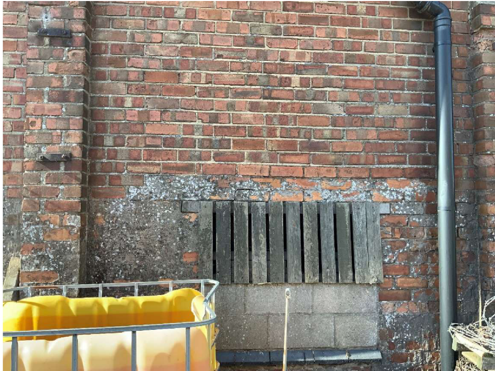
Picture 7 – Minor displacement of brickwork over timber lintel
