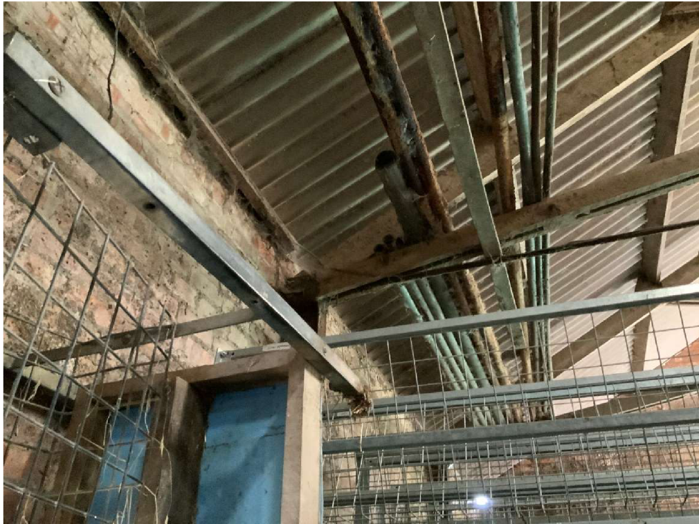
Picture 37 – stored pipes in roof line
