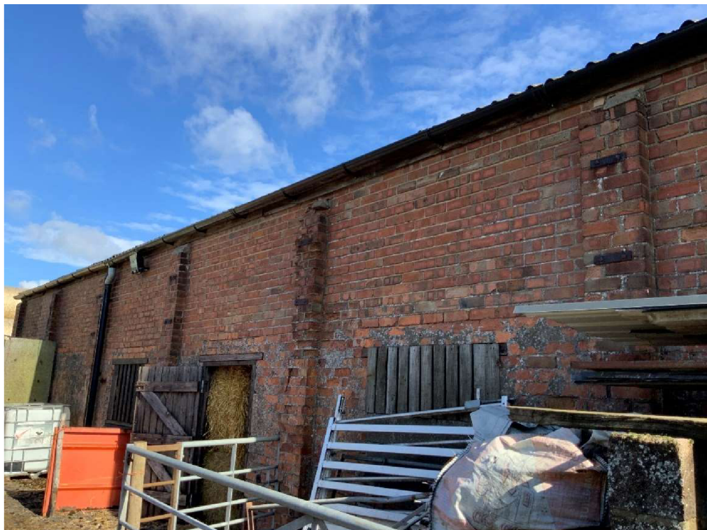
Picture 18 – General view towards north-western corner – note eroded brickwork to central pier to be replaced
