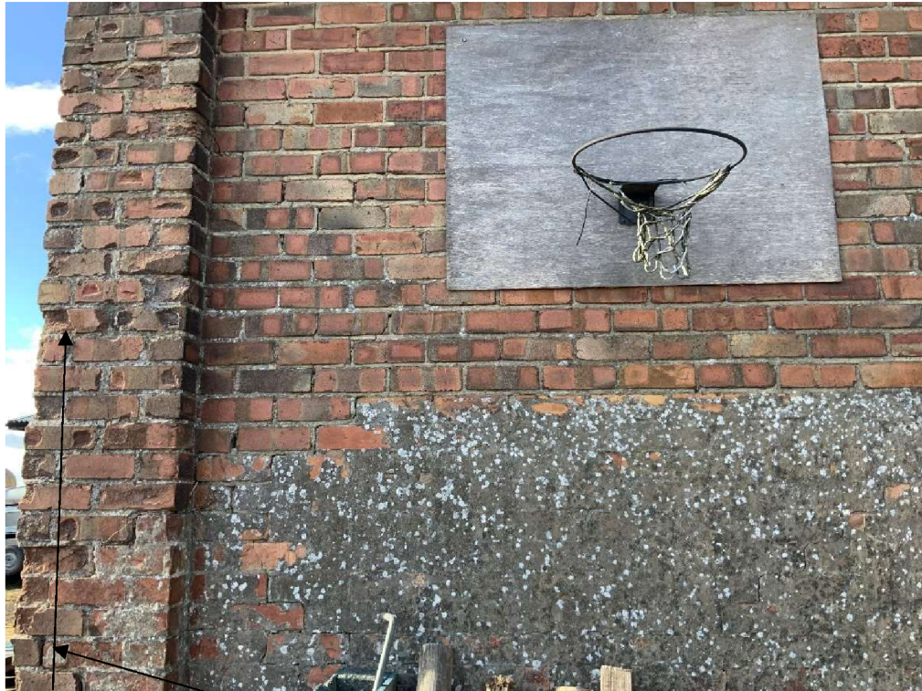
Picture 9 – Brick erosion and impact damage to corner brickwork
