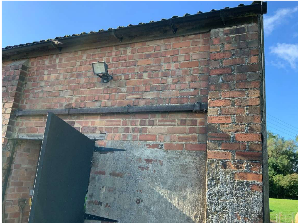
Picture 3 – note lower level thin render and stepped cracking in doorway above shovel handle
