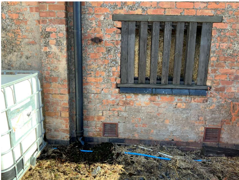
Picture 20 – minor mortar erosion beneath window opening – positive drainage outfall recommended
