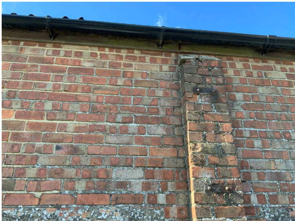
Picture 6 – spalling mortar cap to pier plus light corrosion of strap bolts to internal steel columns
