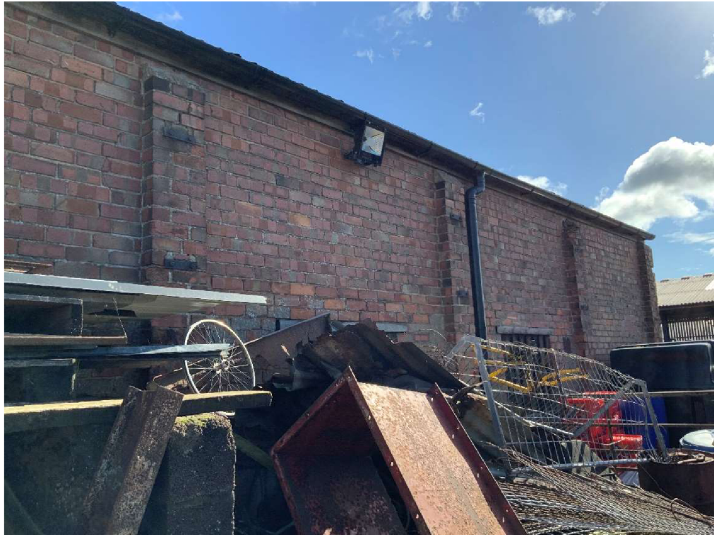
Picture 17 – General view towards south-western corner, note cracked brickwork over centre window opening
