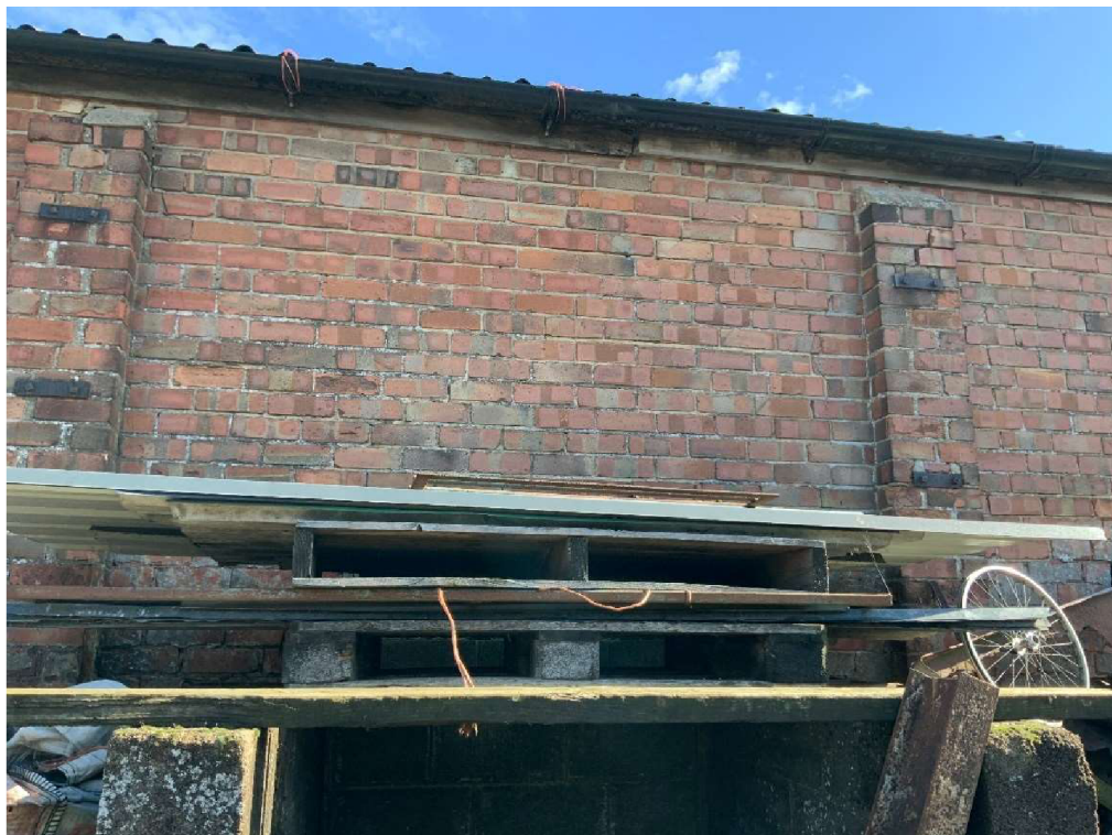
Picture 16 – Mortar coping to pier missing
