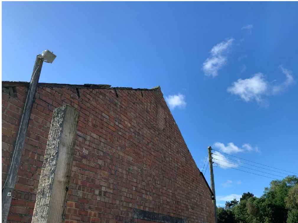
Picture 2 – Exposed verge and purlin protrusion
