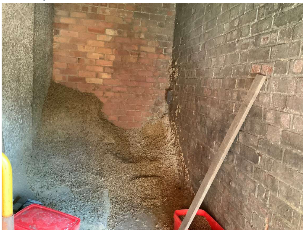
Picture 28 – Stored material in south-eastern corner brickwork which may have caused cracking noted externally
