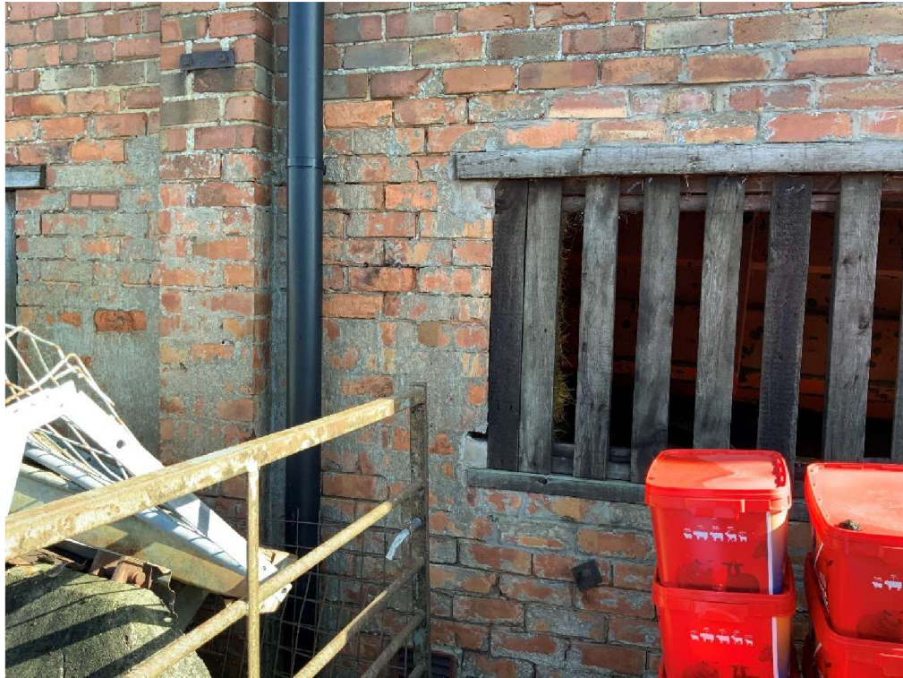
Picture 15 – timber lintels to be replaced as required, minor repointing works
