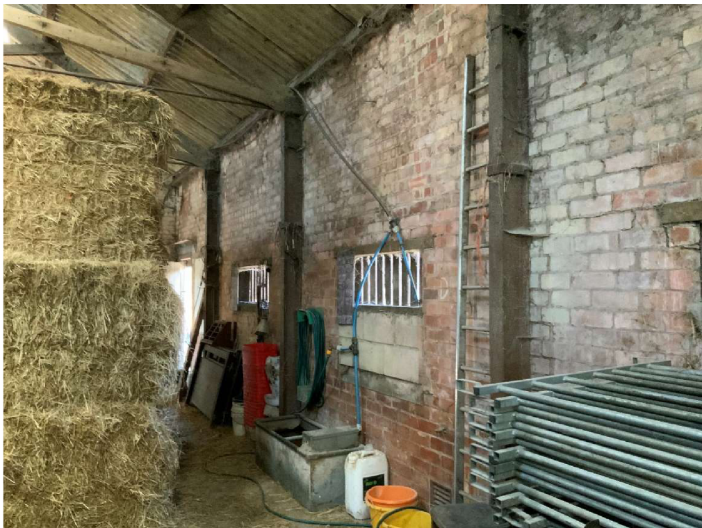
Picture 34 – Note location of strapping bolted through external brick piers at column positions
