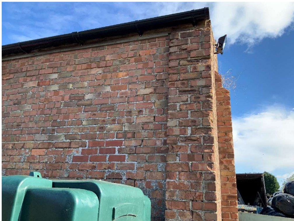
Picture 12 – Cracked and eroded brickwork to corner of barn (south west corner)
