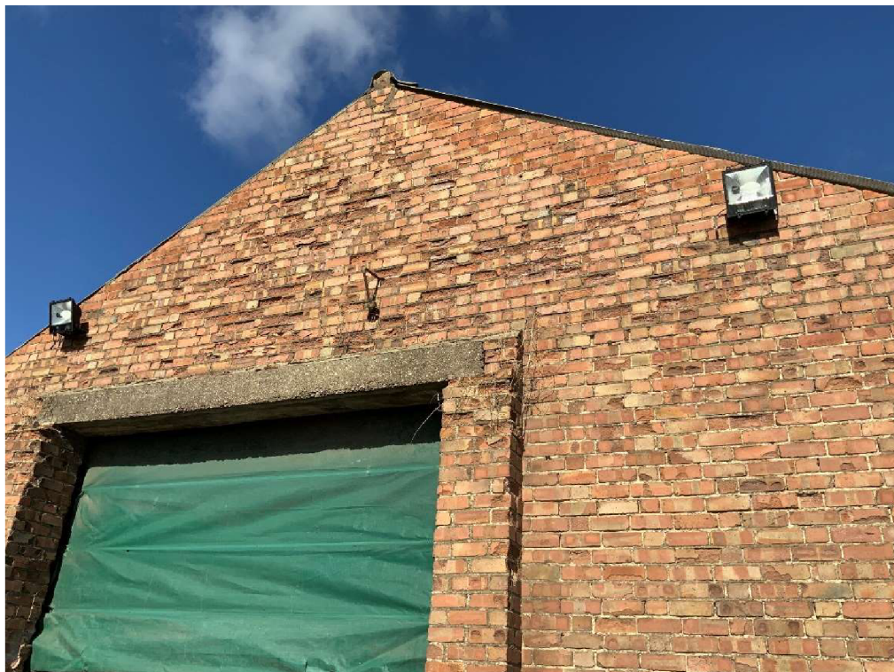
Picture 10 – Eroded gable brickwork and exposed verge
