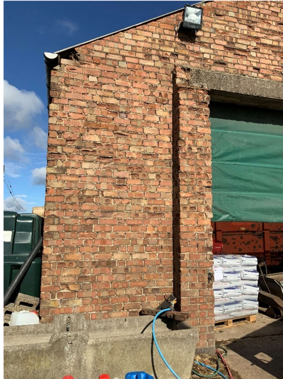
Picture 11 – Missing brickwork at eaves line and eroded brickwork of gable
