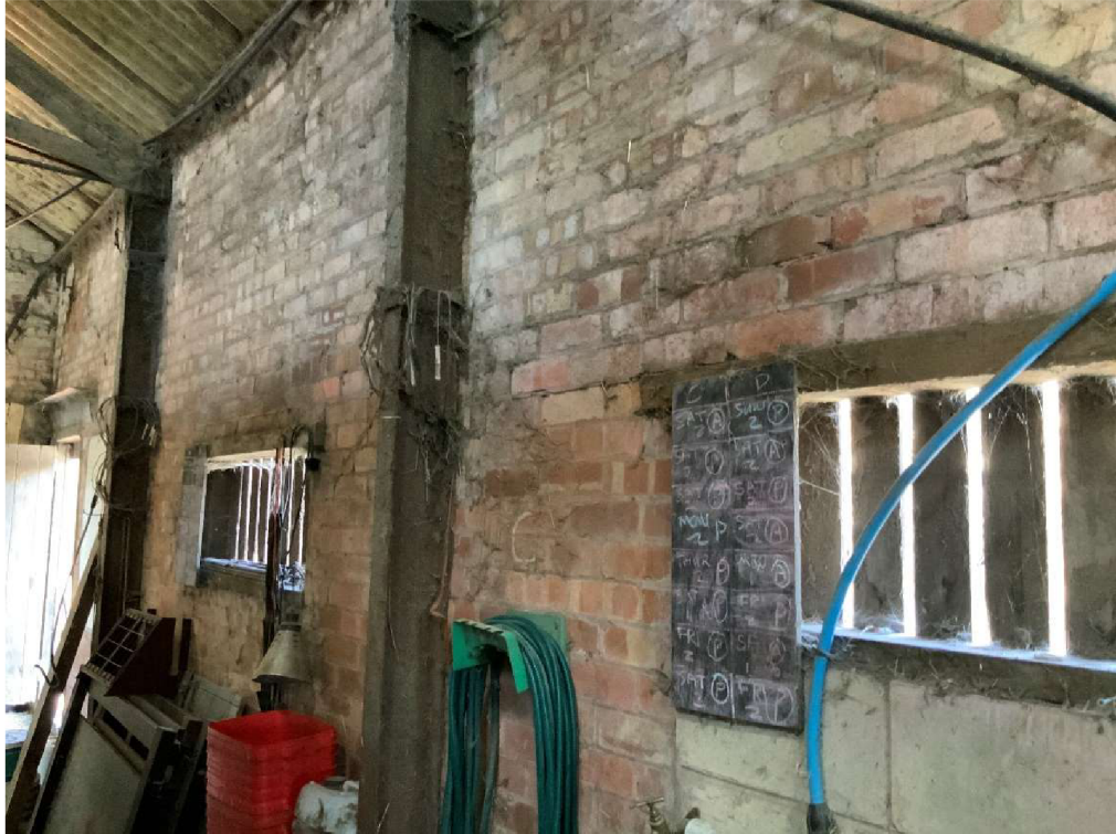
Picture 33 – note change in brickwork approx. 3 courses above window opening
