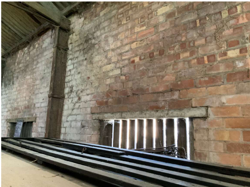
Picture 32 – internal view of cracking over timber lintels
