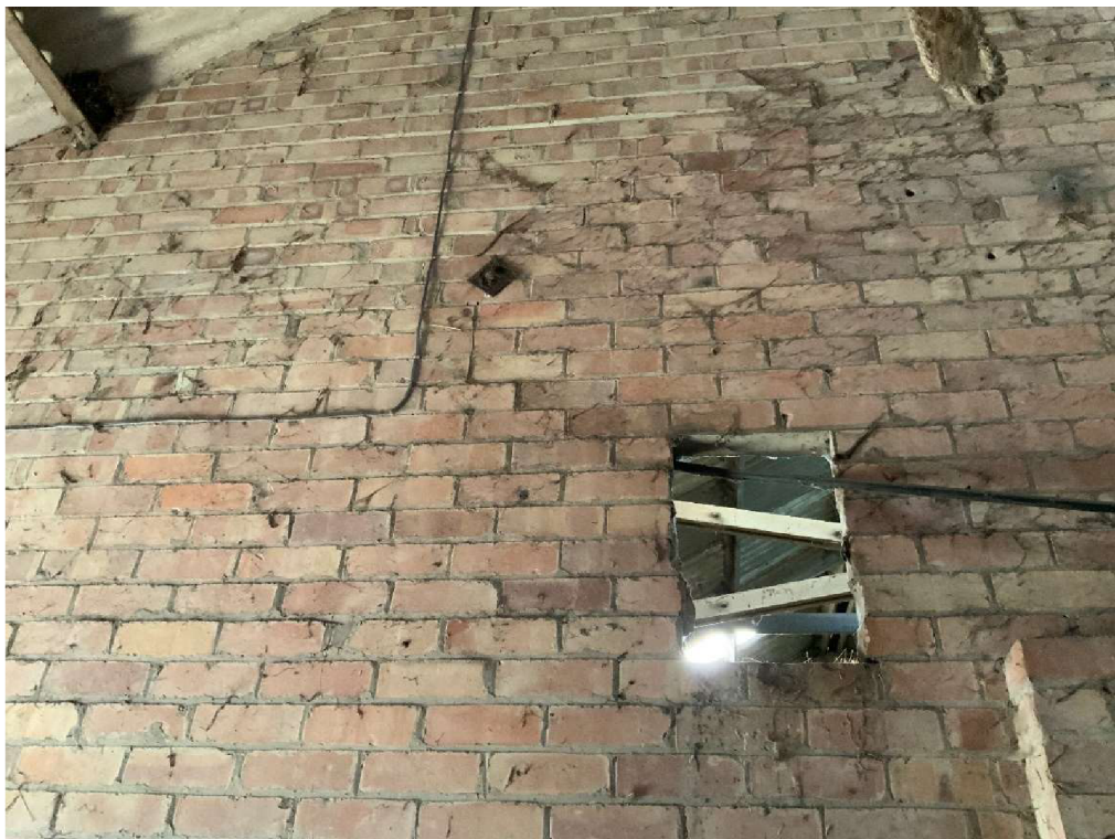
Picture 26 – opening through division wall without lintel over
