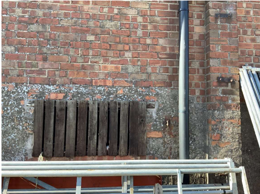
Picture 5 – Minor mortar separation above window lintel
