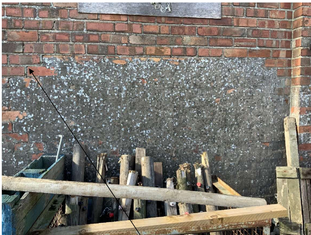
Picture 8 – Slight stepped cracking to left of render line
