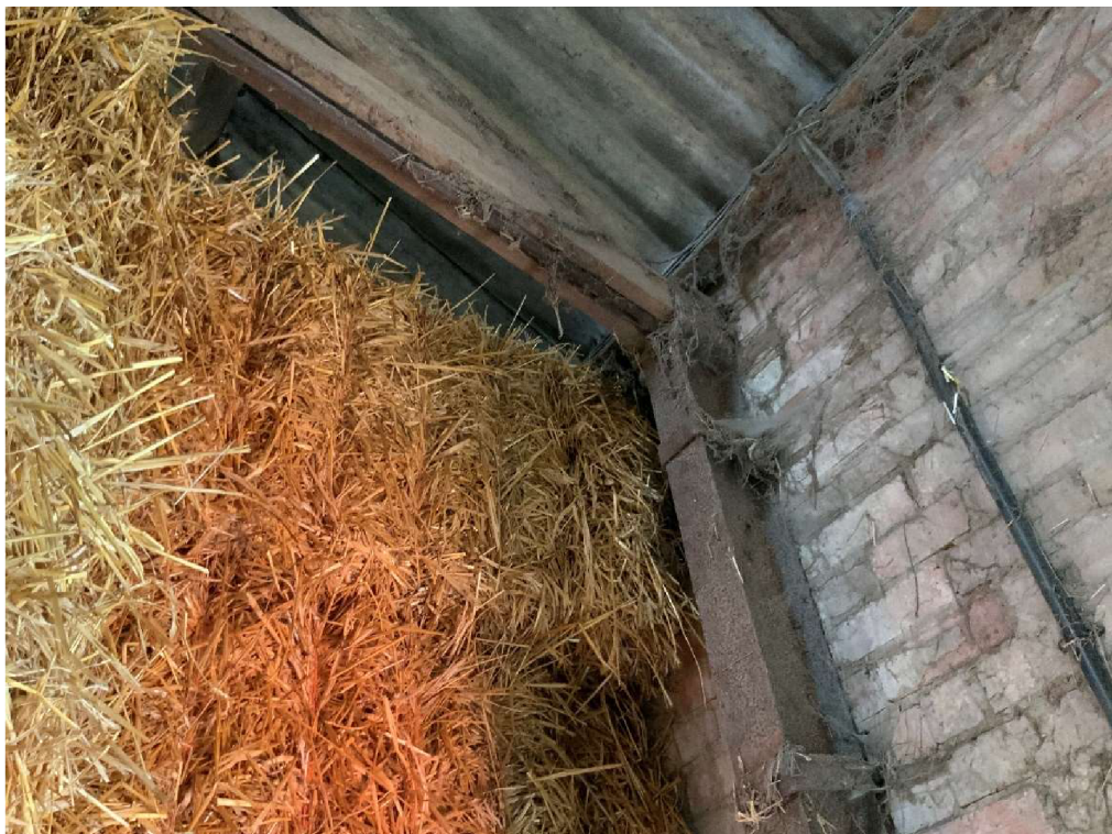
Picture 40 – Open eaves visible as daylight at wall plate
