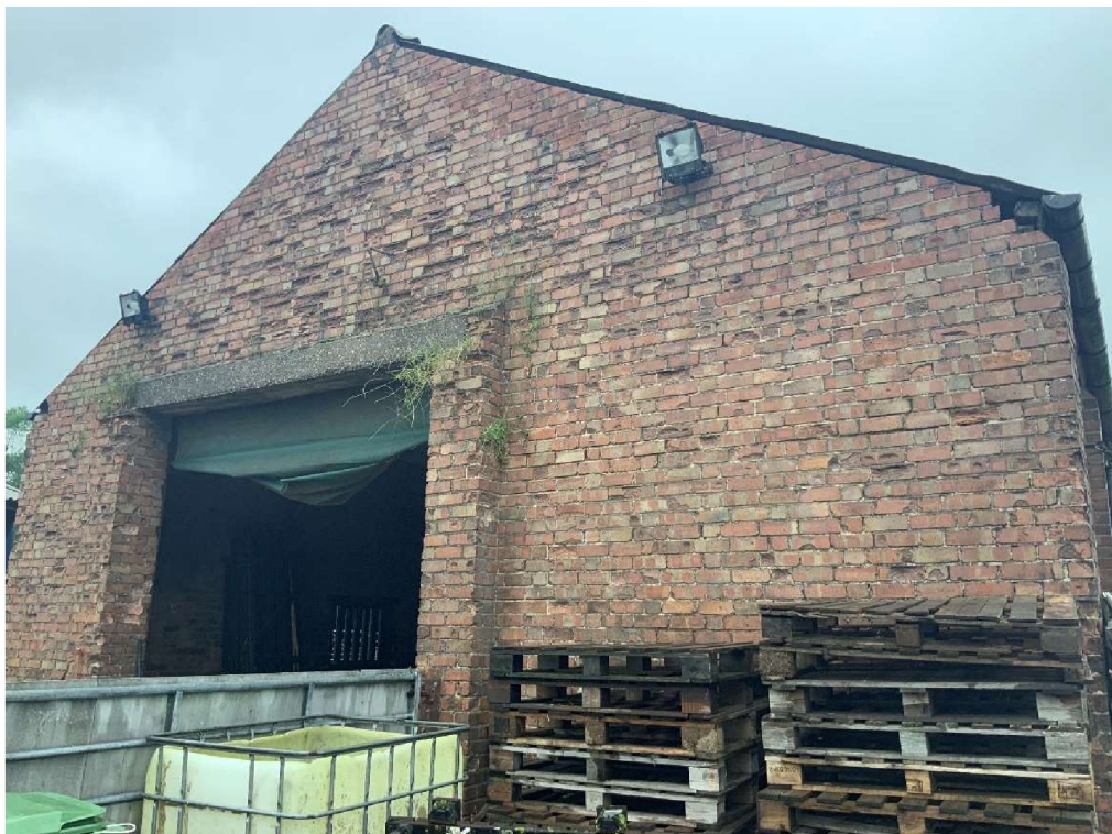
Picture 44 – Southern gable with brick erosion 2023 marginal change and missing eaves bricks
