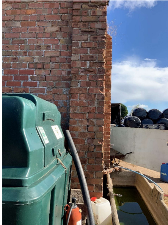
Picture 13 – closer detail of cracked brickwork to corner
