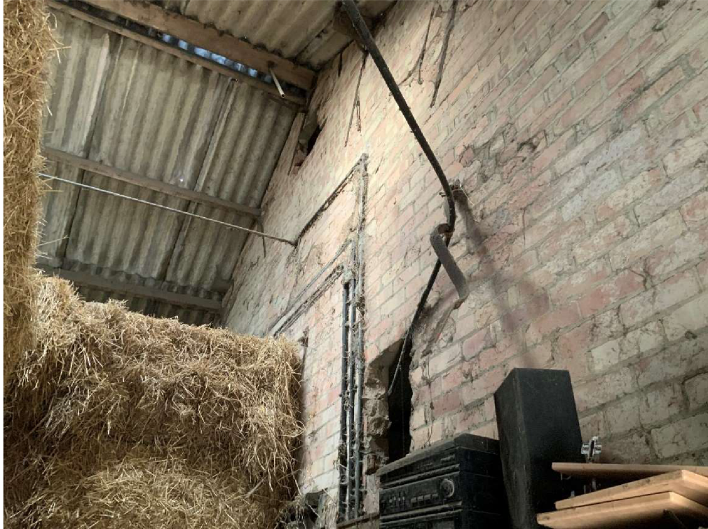
Picture 39 – hole through wall with no lintel – visible daylight at roof vent position (adequate)
