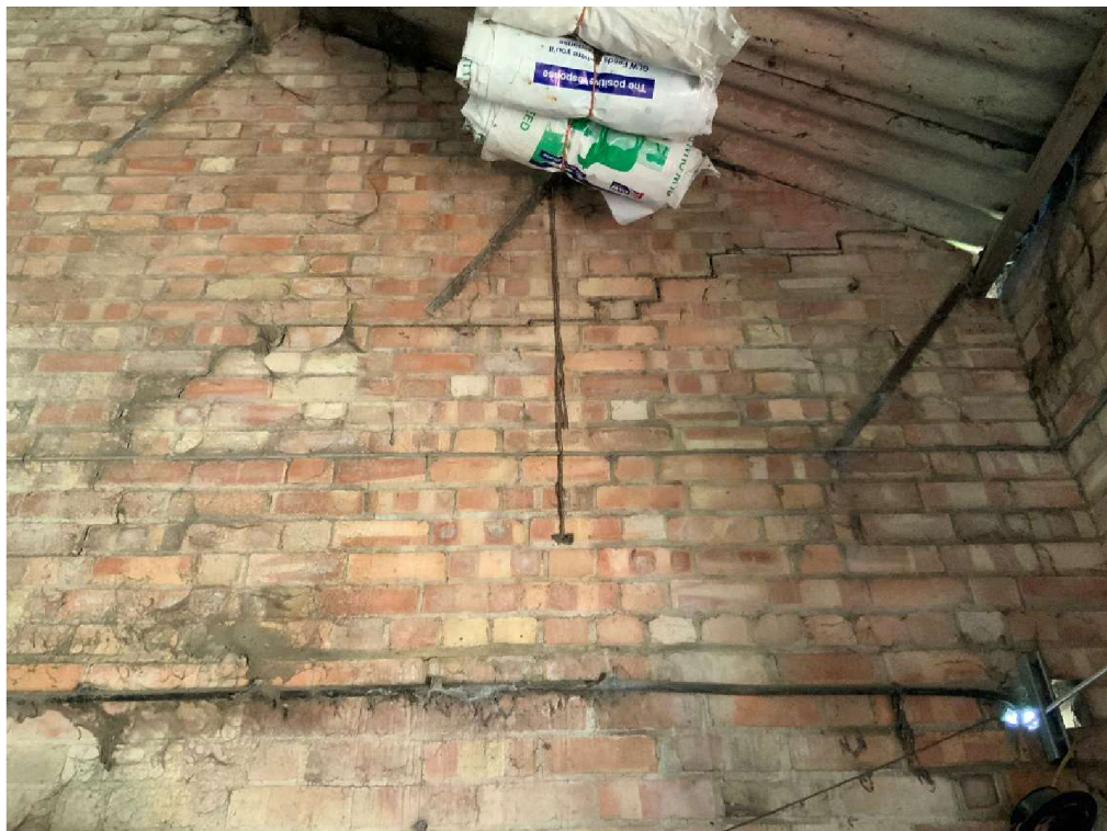
Picture 24 – Stepped cracking to north east corner brickwork to be raked out and repointed
