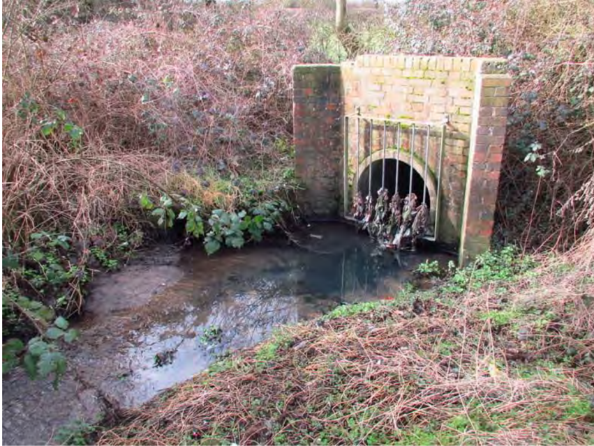
Plate 1 – Start of the Earl Shilton Brook – surface water outlet – note rag debris
