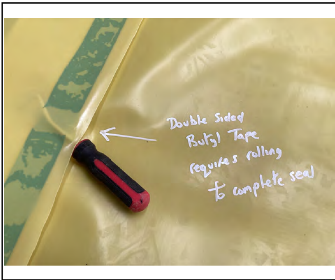
View of un-sealed lap joint requiring further pressure to complete seal (1)
