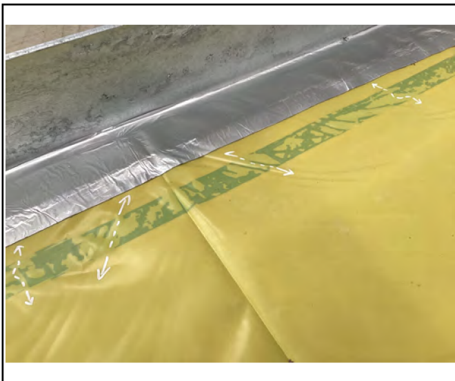
View of un-sealed lap joint requiring further pressure to complete seal (2)
