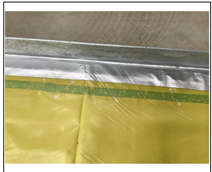
Un-sealed lap joint (2) remediated following further pressure application
