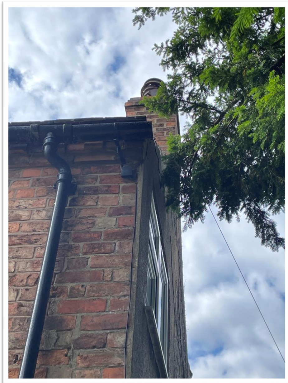
Fig 2. Picture showing crown near building.
