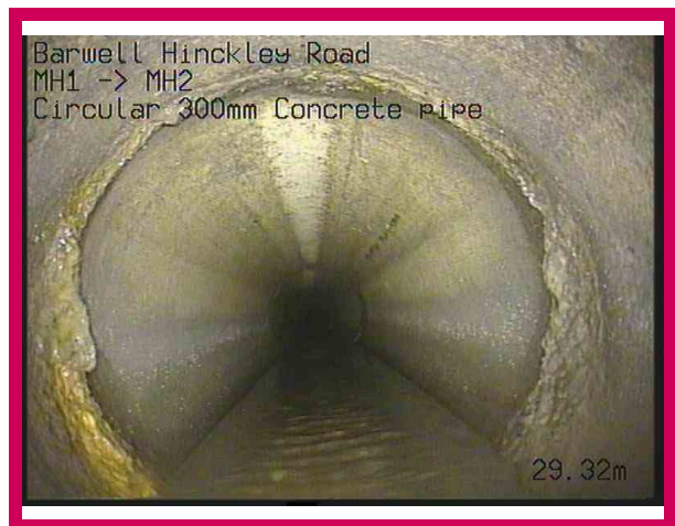
MH1X_caa4ccd6-a175-469f-9445-378d2495e79a_20230512_092838_343.jpg, 00:04:27, 29.31 m Attached deposits, encrustation at joint from 12 o'clock to 12 o'clock, 5% cross-sectional area loss, start
