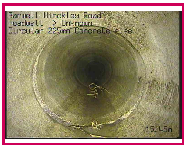
HeadwallZ_ed0df475-4ebc-498f-b62e-c4c11c447984_20230608_101406_030.jpg, 00:02:30, 15.45 m Roots, fine at joint, start
