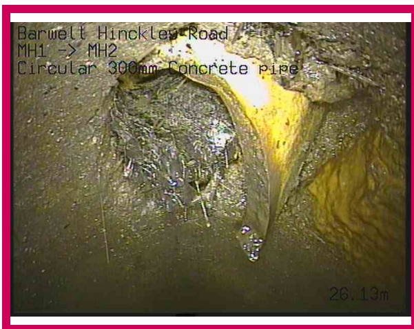
MH1X_9d364977-05eb-40c5-8a1d-4b2cbe5c1326_20230512_092742_945.jpg, 00:03:46, 26.13 m Connection defective, connecting pipe is blocked at 01 o'clock, diameter: 150mm
