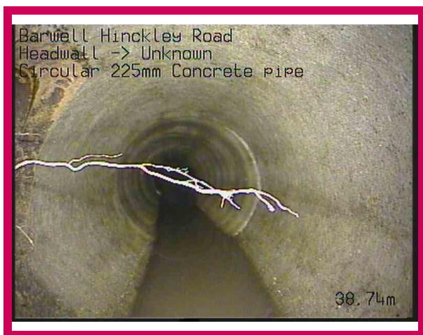
HeadwallA_1a61a5c5-41b7-47a5-a858-f0ddada7ab86_20230608_104613_162.jpg, 00:04:36, 38.74 m Junction at 11 o'clock, diameter: 100mm
