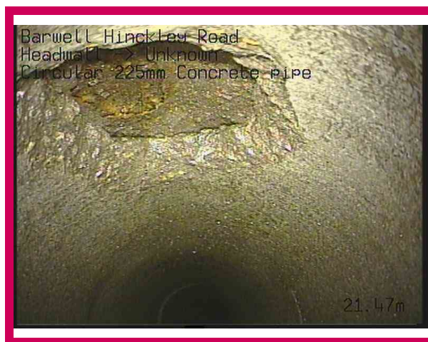
HeadwallZ_7866e841-7100-4af3-8475-b18f6978f9f6_20230608_101520_678.jpg, 00:03:34, 21.47 m Hole in drain or sewer from 11 o'clock to 12 o'clock
