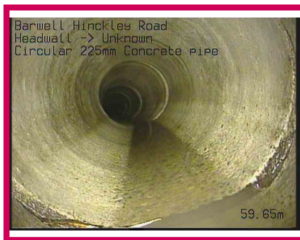
HeadwallA_247d0fcd-3474-4e02-8490-c9ee06e1604d_20230608_134839_398.jpg, 00:06:17, 59.65 m Roots, fine at joint
