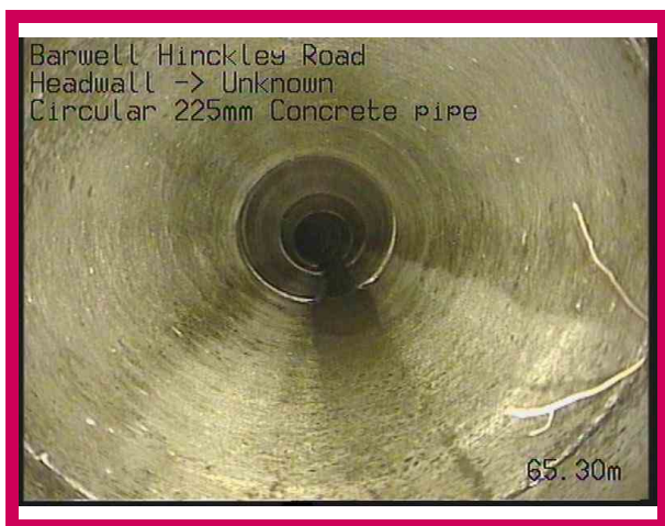
HeadwallA_b0145eaf-9605-414f-9f97-1fa380cf1c8b_20230608_134932_957.jpg, 00:00:00, 65.30 m Roots, fine at joint
