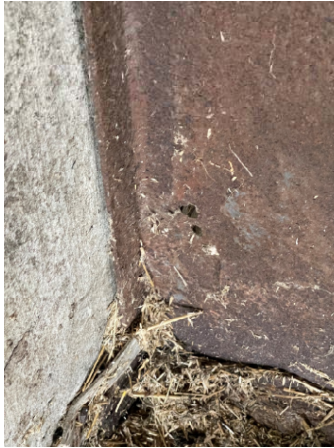
Figure 13: Section loss of column
