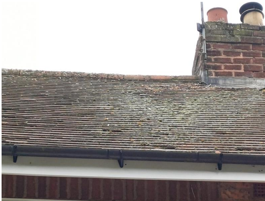
Photograph 4: Raised tiles at the rear of the building.
