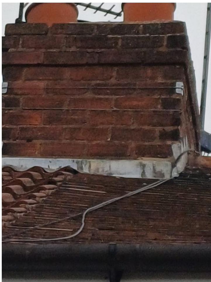
Photograph 5: Gap between the lead flashing and tiles at the front of the building.
