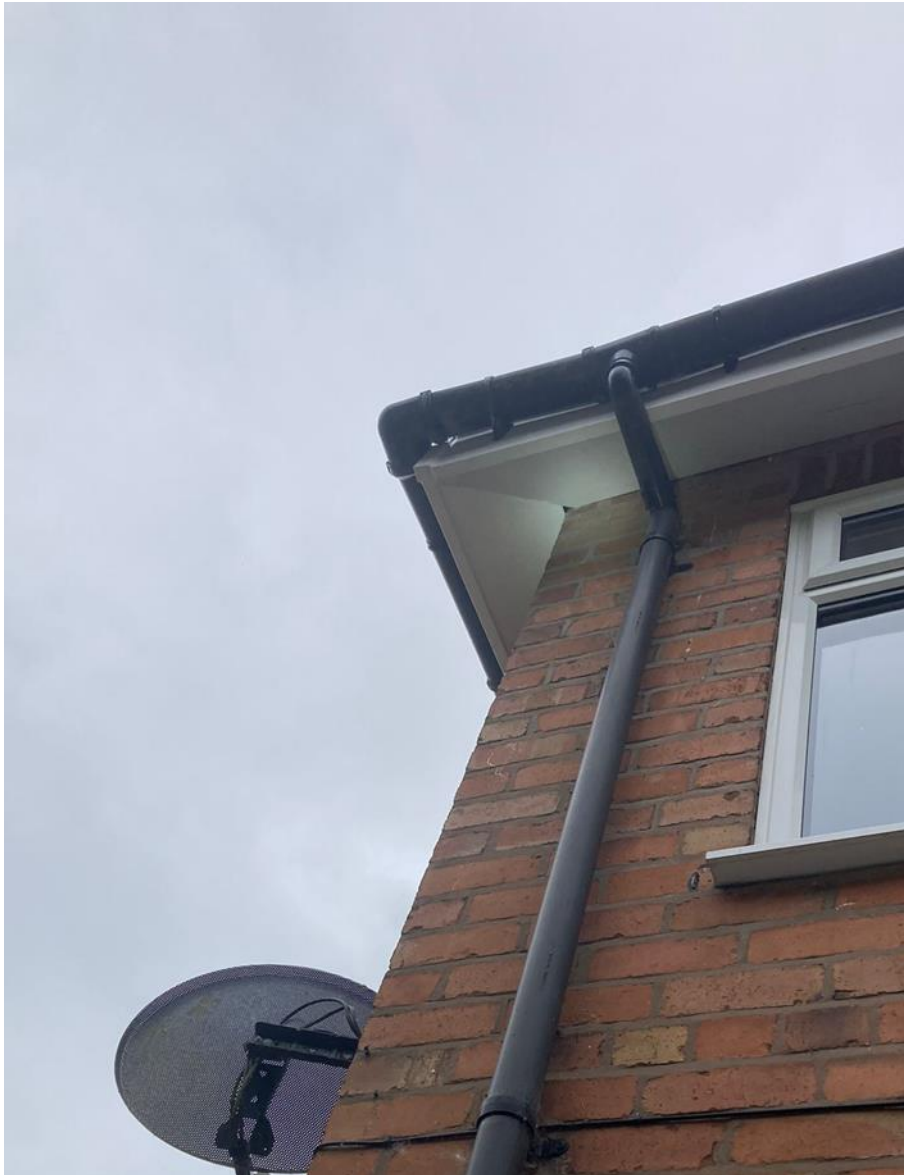
Photograph 6: Access point in the soffit directly above the bird droppings.
