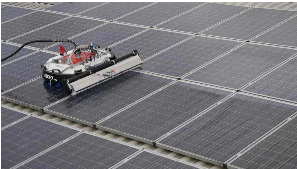
D. 003 – Cleaning of modules by Robot example
