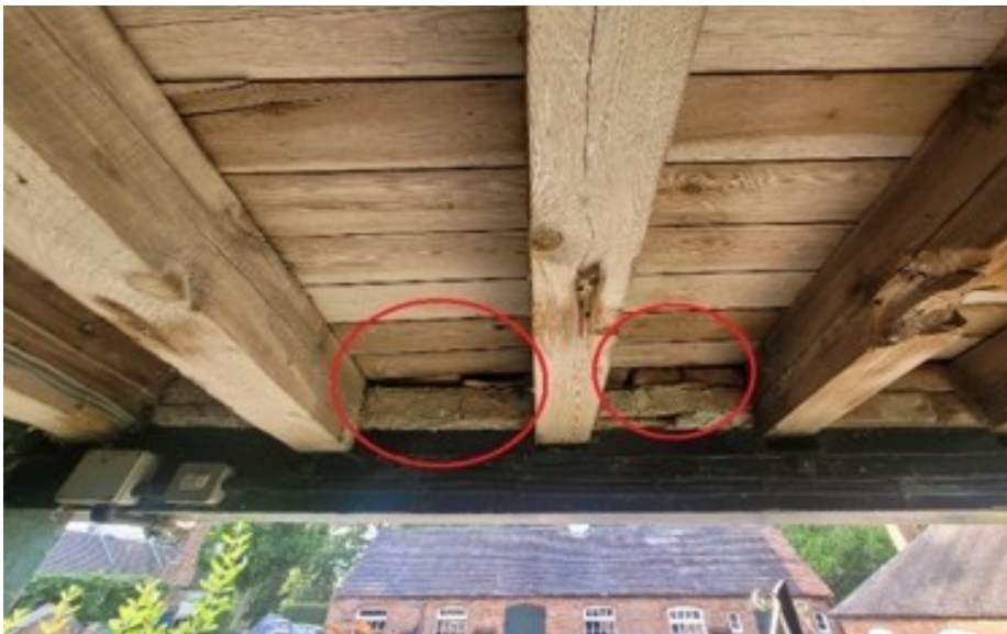
Figure 12 Gaps in brickwork at eaves in center of B2
