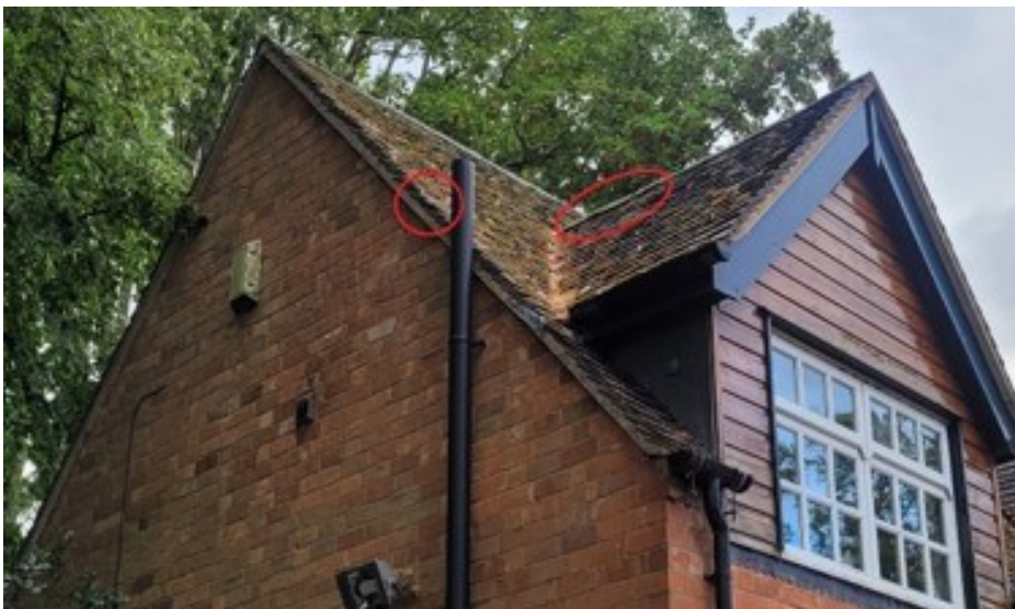
Figure 4 Lifted tiles and ridge southern elevation
