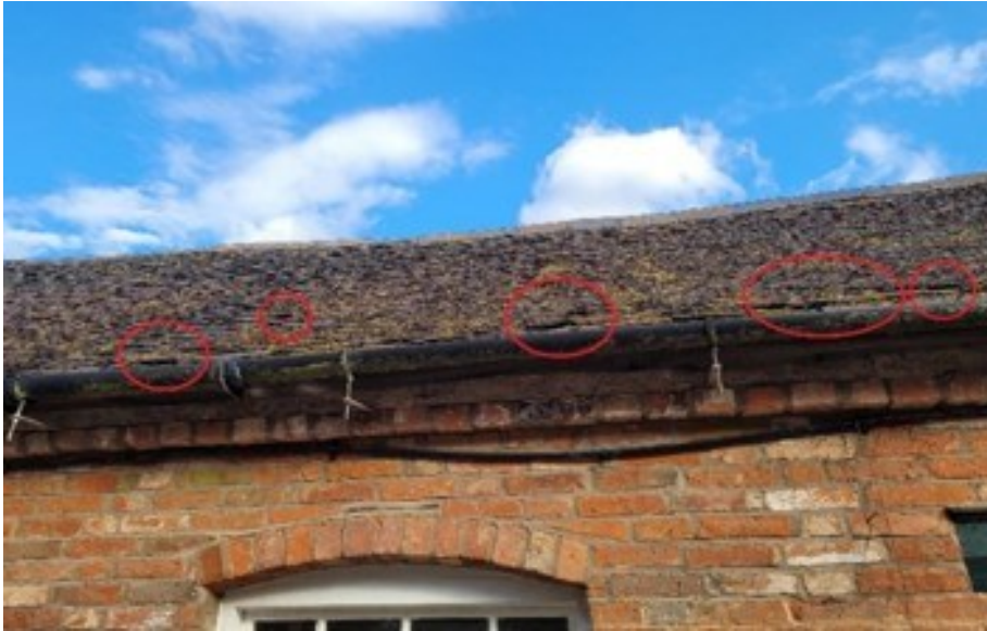
Figure 11 Lifted tiles B2
