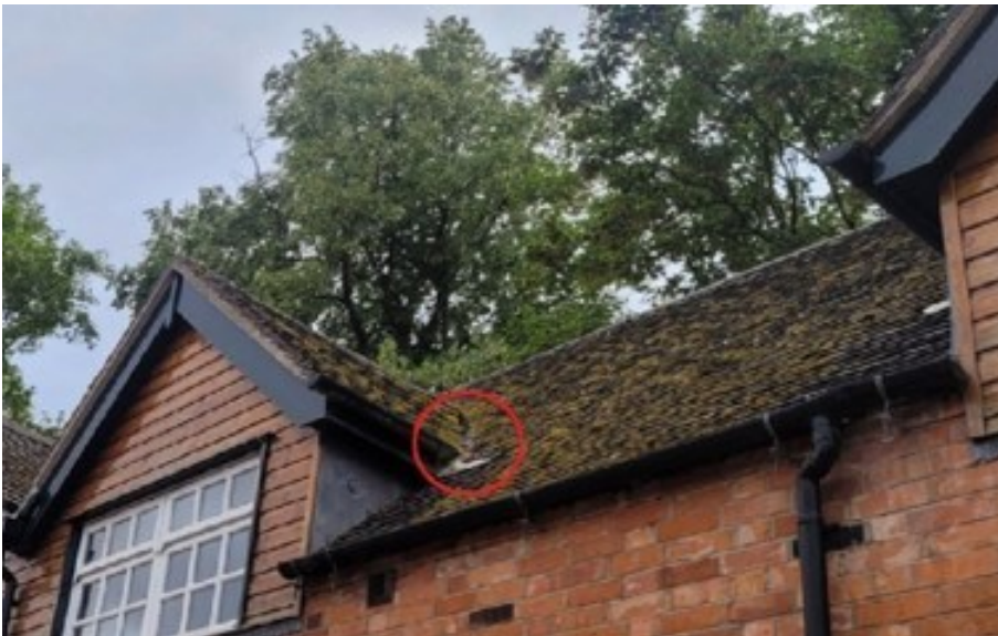
Figure 6 Lifted lead flashing on junction facing east
