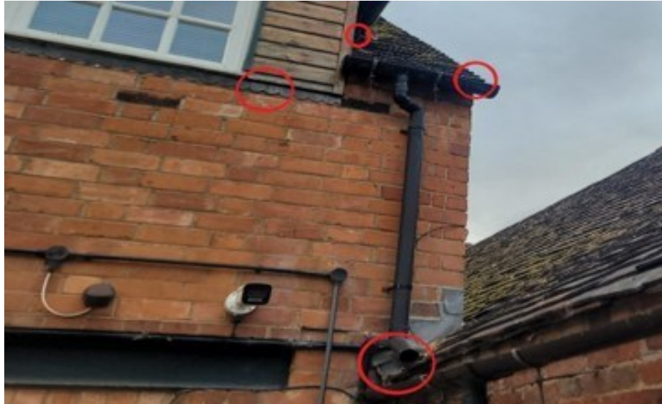
Figure 7 Lifted lead flashing, tiles and trim
