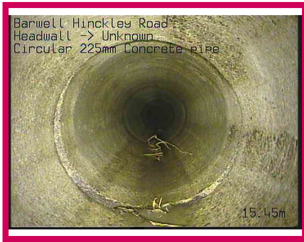
HeadwallZ_ed0df475-4ebc-498f-b62e-c4c11c447984_20230608_101406_030.jpg, 00:02:30, 15.45 m Roots, fine at joint, start
