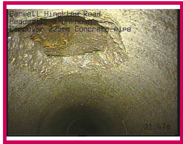
HeadwallZ_7866e841-7100-4af3-8475-b18f6978f9f6_20230608_101520_678.jpg, 00:03:34, 21.47 m Hole in drain or sewer from 11 o'clock to 12 o'clock
