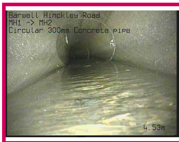
MH1X_9358778a-2684-4085-95bd-070cae35a578_20230512_092347_170.jpg, 00:00:38, 4.53 m Settled deposits, hard or compacted, 5% cross-sectional area loss, start
