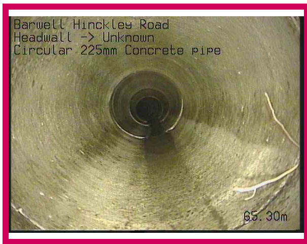
HeadwallA_b0145eaf-9605-414f-9f97-1fa380cf1c8b_20230608_134932_957.jpg, 00:00:00, 65.30 m Roots, fine at joint
