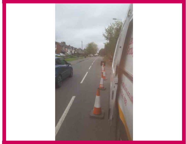
Further works will need TM (2)
