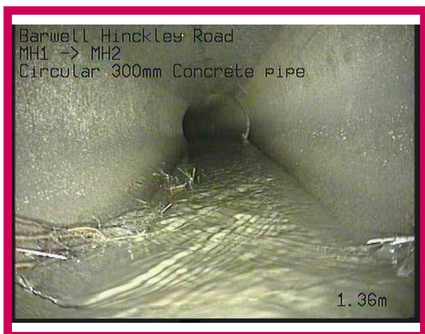
MH1X_be1794be-3572-4021-a4f4-c6ea53cc6a12_20230512_092320_558.jpg, 00:00:14, 1.36 m Roots, fine at joint, start
