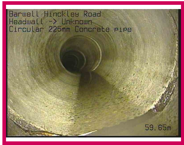
HeadwallA_247d0fcd-3474-4e02-8490-c9ee06e1604d_20230608_134839_398.jpg, 00:06:17, 59.65 m Roots, fine at joint
