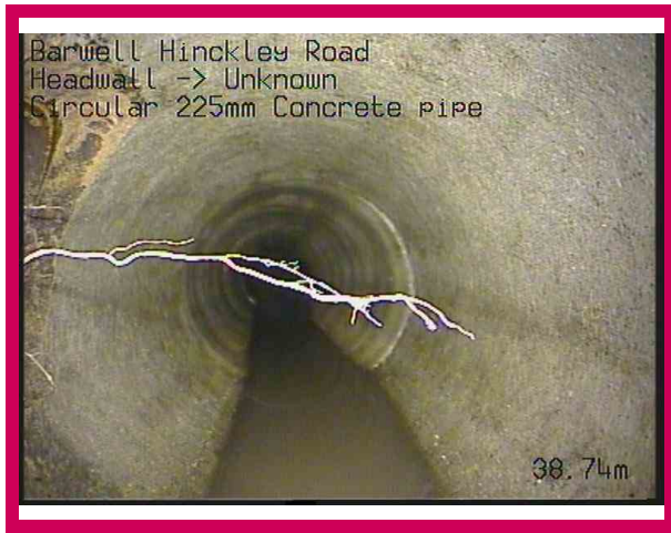
HeadwallA_1a61a5c5-41b7-47a5-a858-f0ddada7ab86_20230608_104613_162.jpg, 00:04:36, 38.74 m Junction at 11 o'clock, diameter: 100mm
