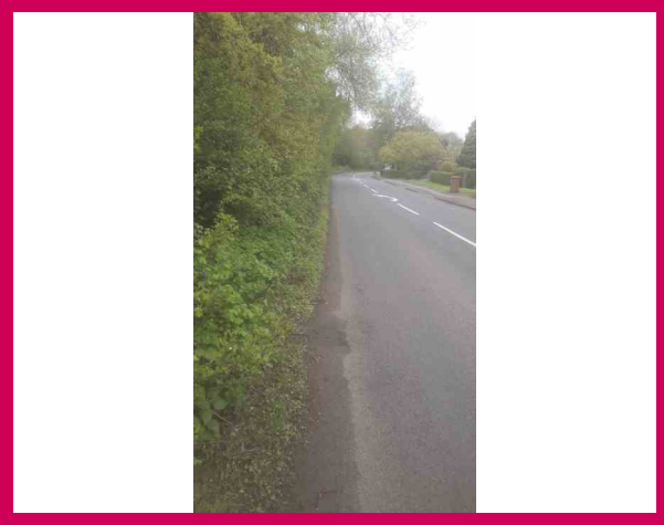
Further works will need TM (1)
