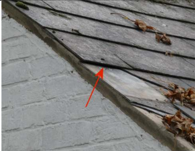
Photograph 13. Slip tile on the 2 section at the north-west end of the Farmhouse
