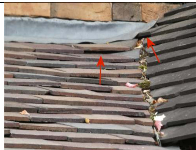
Photograph 35. Example of openings under tiles on the single-storey section at the south-east end of The Granary
