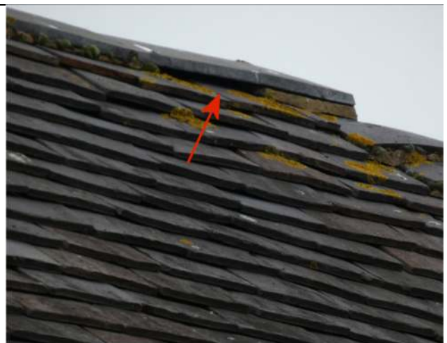
Photograph 34. Example of an opening under a ridge tile on the south-east facing roof pitch of the Granary
