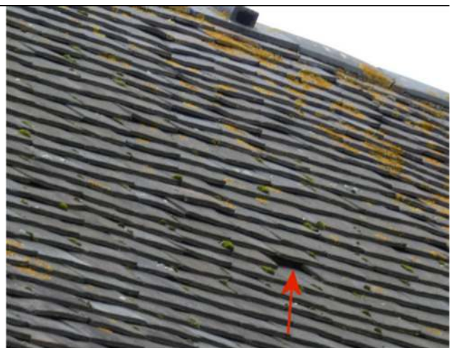
Photograph 36. Example of a missing tile on the north-east facing roof pitch of The Granary
