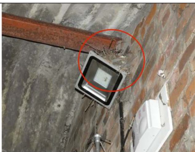
Photograph 61. Pigeons nest within the interior of Barn 5
