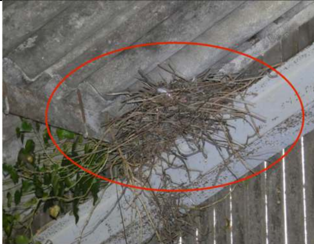
Photograph 63. Pigeons nest within the interior of Barn 17
