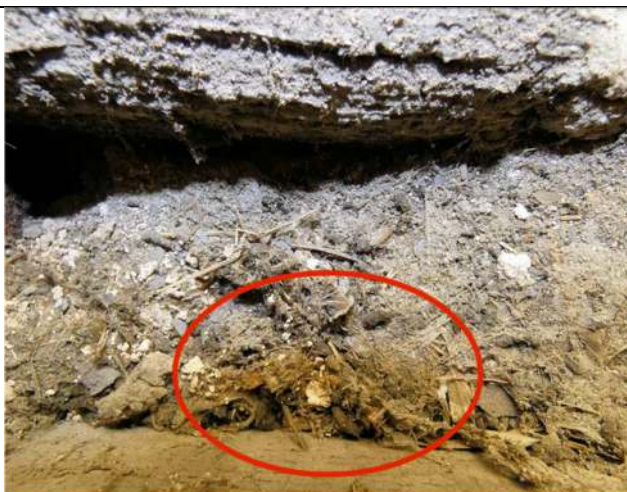
Photograph 23. Old bat droppings at the edge of the enclosed roof void in the south-east half of the main part of the Farmhouse
