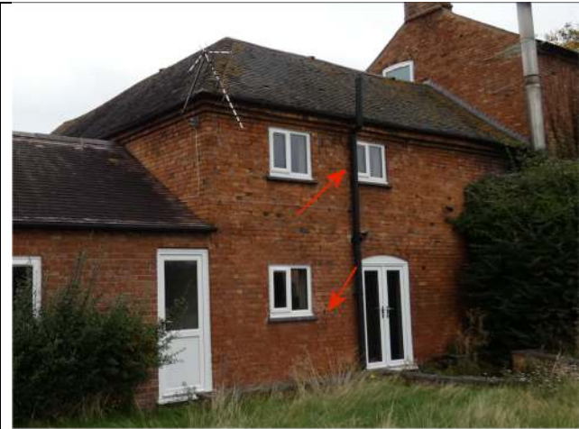
Photograph 37. Location of crevices in the brickwork on the north-east side of The Granary
