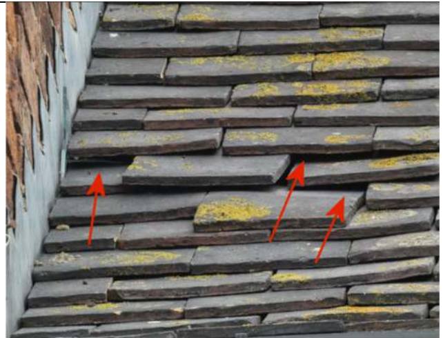
Photograph 32. Example of openings under tiles on the roof of The Granary (south-west facing roof pitch)
