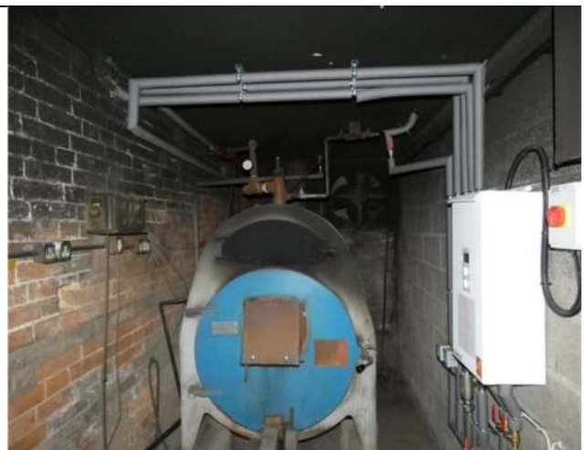
Photograph 40. The interior of the boiler room within The Granary
