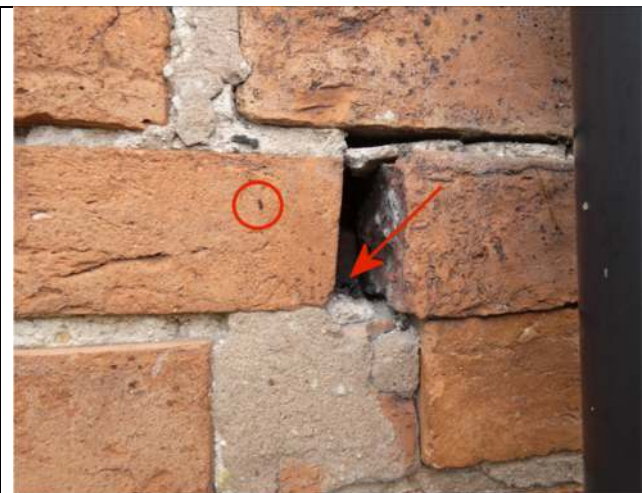
Photograph 39. Bat droppings in a crevice in the brickwork on the north-east side of The Granary
