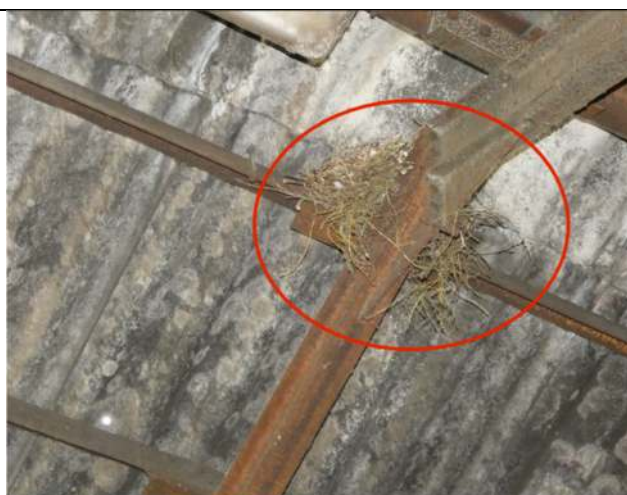
Photograph 62. Pigeons nest within the interior of Barn 8
