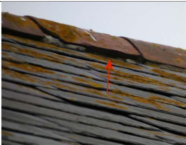
Photograph 15. Further example of a possible opening under a ridge tile on the north-east facing roof pitch of the main part of the Farmhouse
