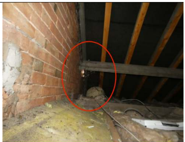
Photograph 42. Active wasp nest within the enclosed roof void within the single-storey section at the north-east end of The Granary
