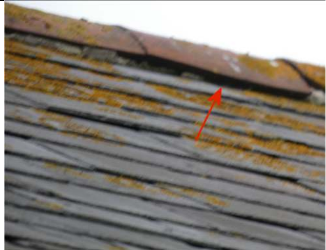
Photograph 14. Possible opening under a ridge tile on the north-east facing roof pitch of the main part of the Farmhouse
