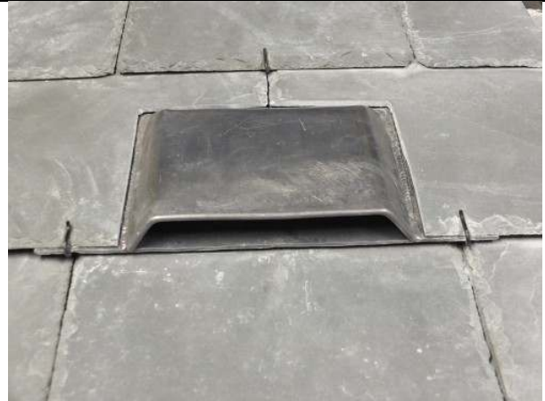
Photograph 64. Example of a bat access slate
