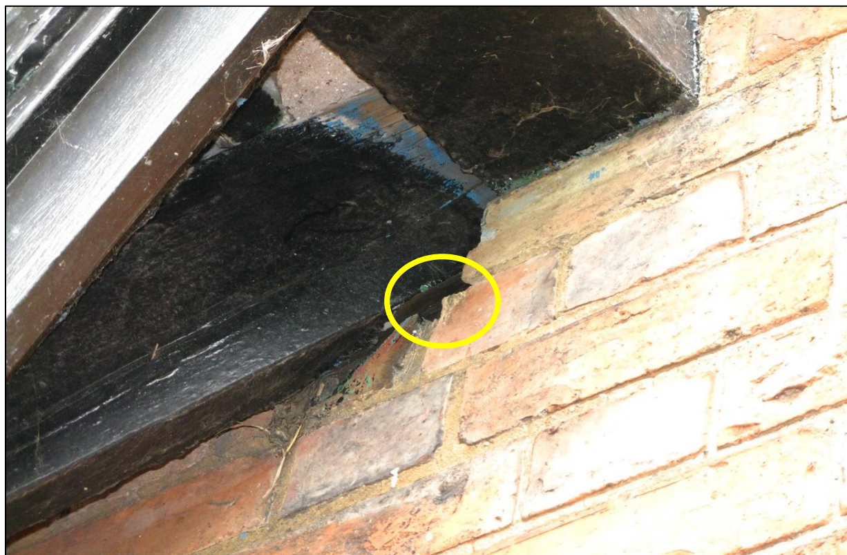
Photograph 12: Gap between end of purlin and brickwork on southern aspect
