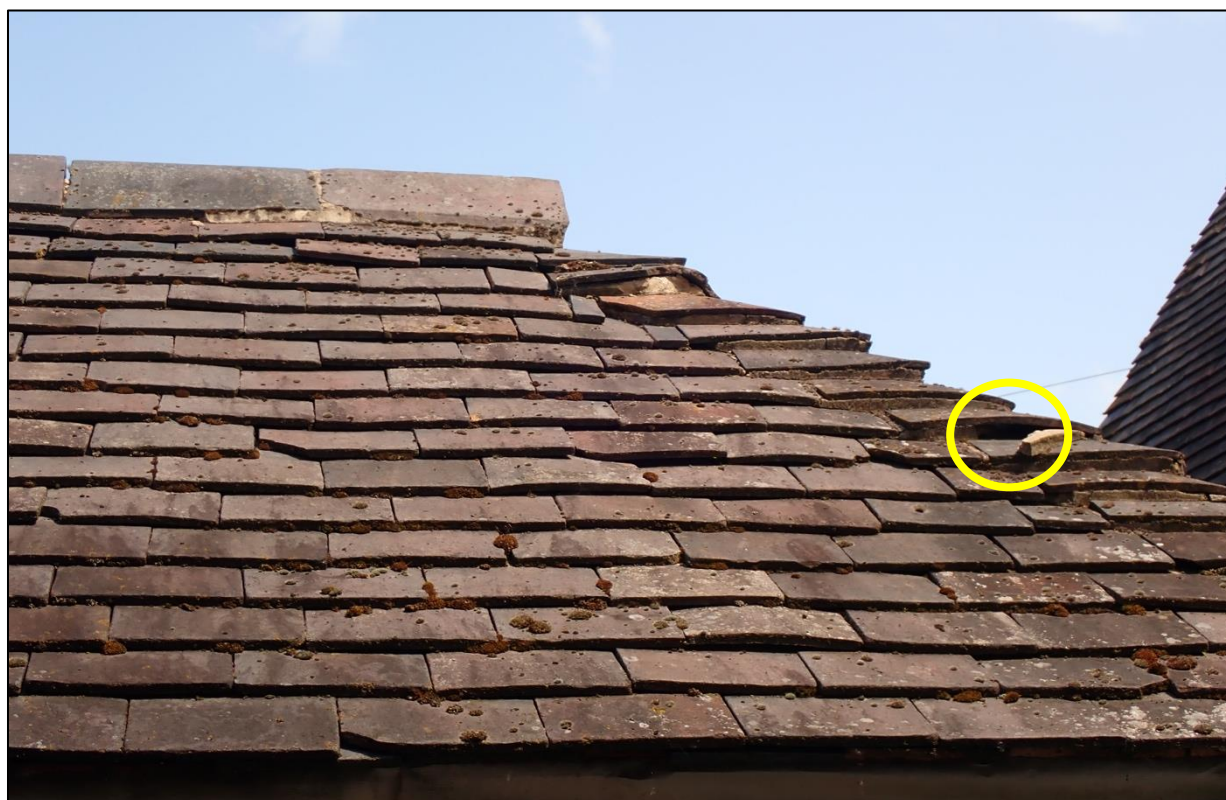
Photograph 14: Gap under hip tile and raised roof tiles on southern aspect of outbuilding
