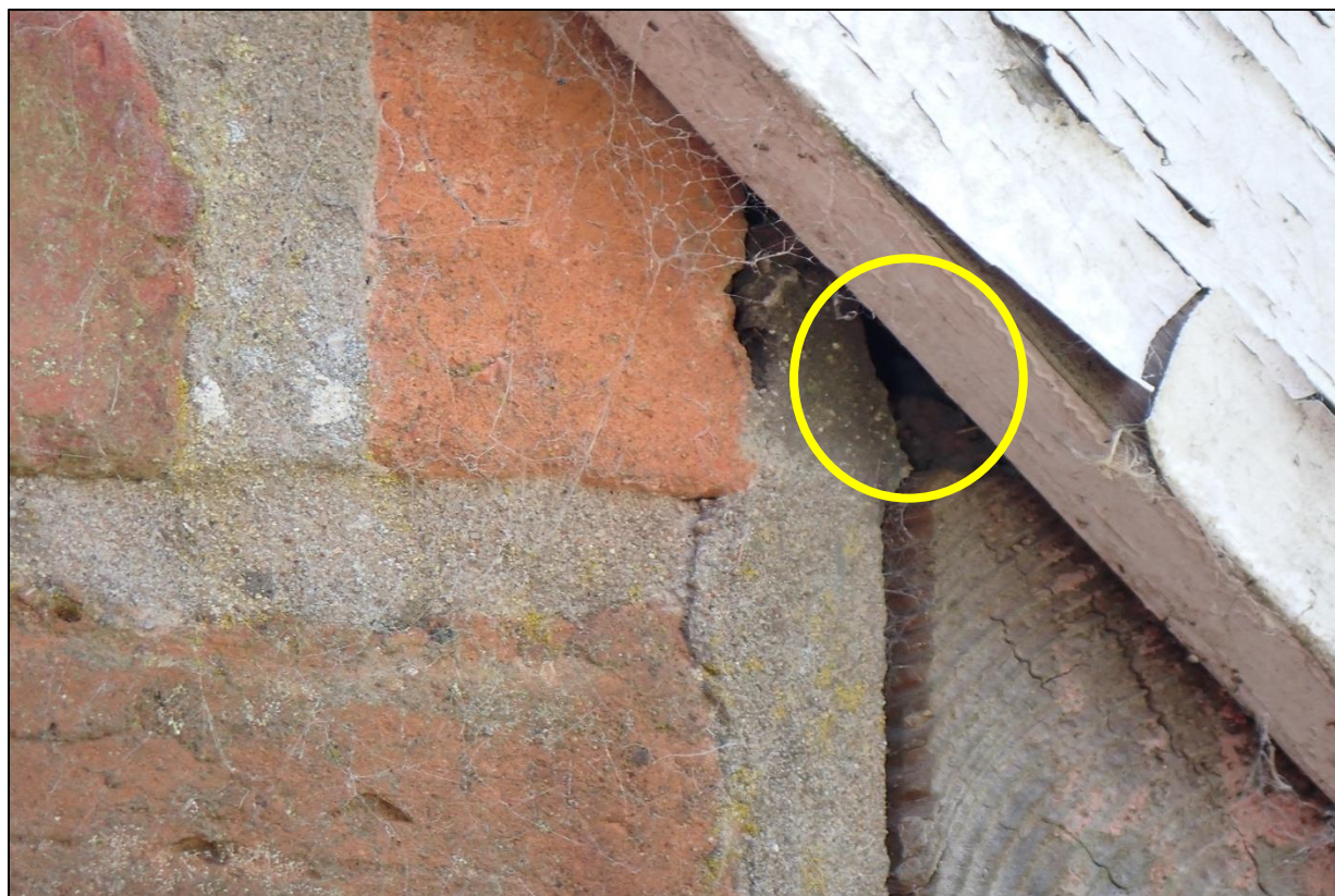
Photograph 16: Gap under fascia board on western aspect of outbuilding
