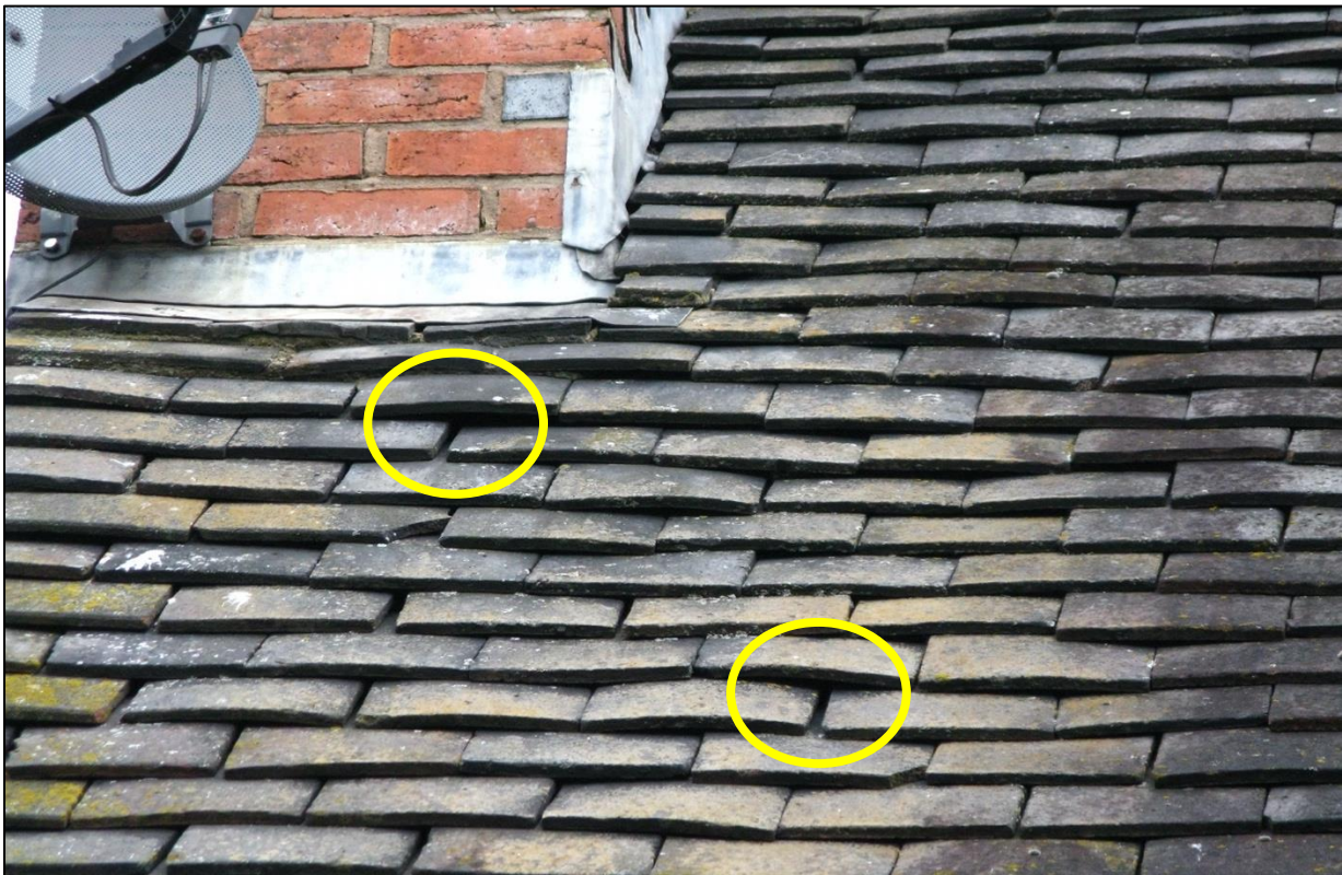
Photograph 9: Gaps under lead flashing surrounding chimney on southern aspect
