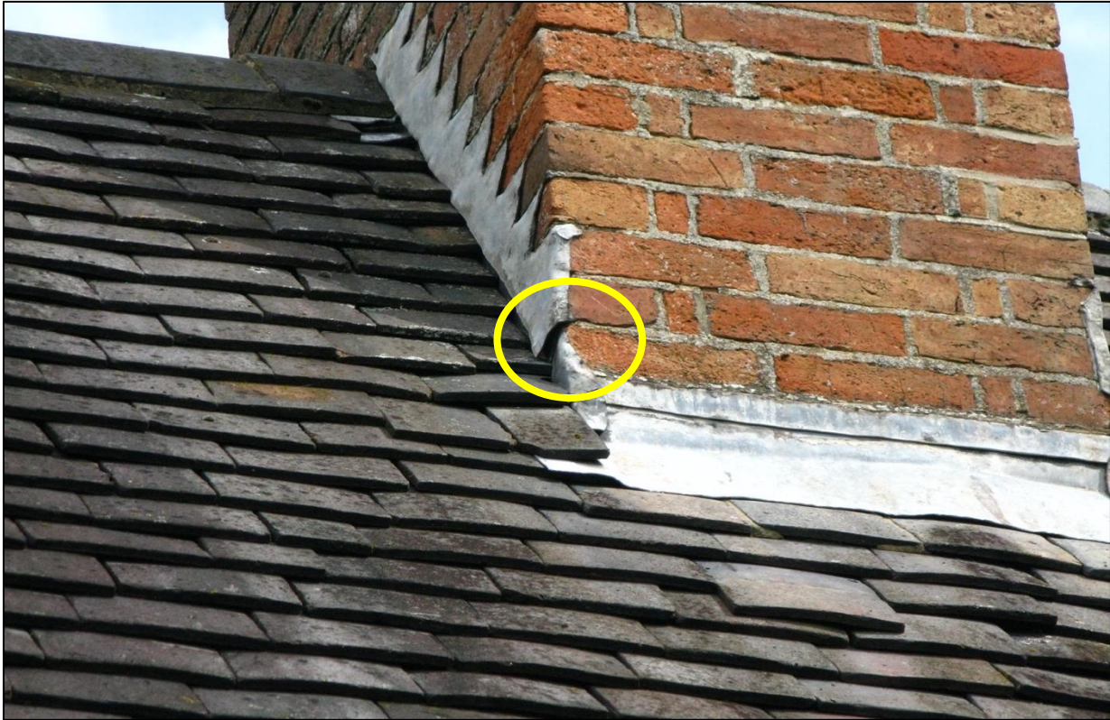
Photograph 10: Gaps under lead flashing surrounding chimney on southern aspect
