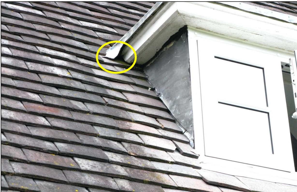
Photograph 11: Gap under lead cladding on dormer on southern aspect
