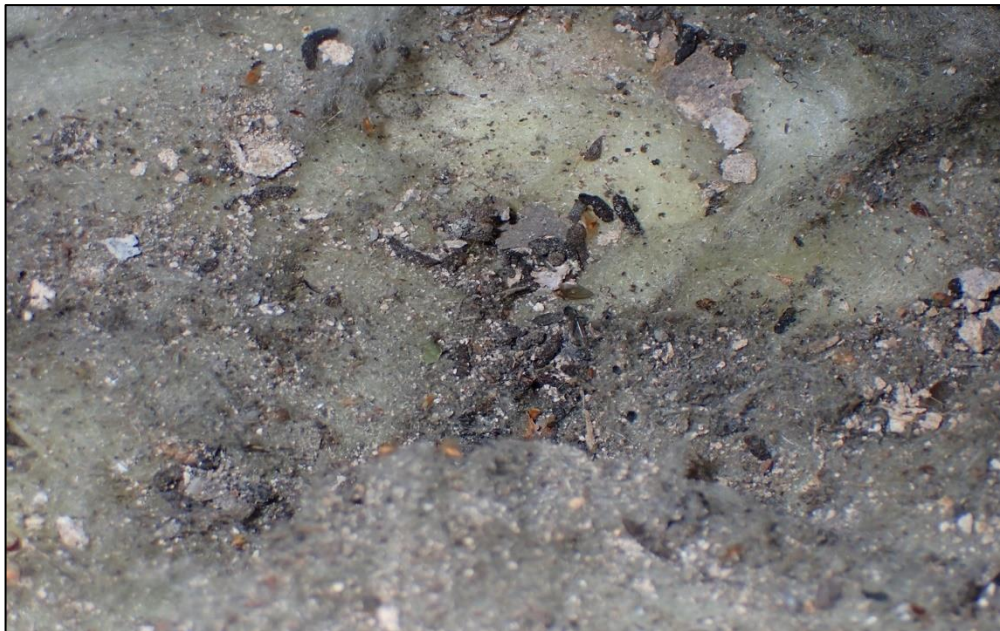
Photograph 7: Scattered Whiskered bat droppings identified on top of the fibre-glass floor covering within the internal roof void of the main two-storey building
