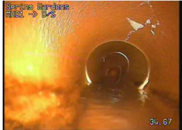
7_MH01_Downstream_DS.jpg, 00:06:20, 34.67 m Crack, longitudinal at 12 o'clock
