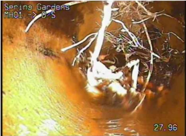
6_MH01_Downstream_DS.jpg, 00:04:37, 27.93 m Roots, tap at joint
