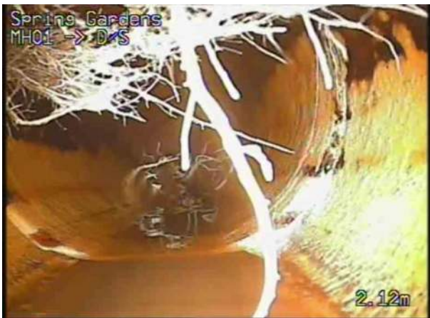
4_MH01_Downstream_DS.jpg, 00:00:49, 2.21 m Crack, circumferential at joint from 1 o'clock to 5 o'clock
