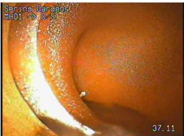
8_MH01_Downstream_DS.jpg, 00:06:41, 37.11 m Line deviates left, Sharp
