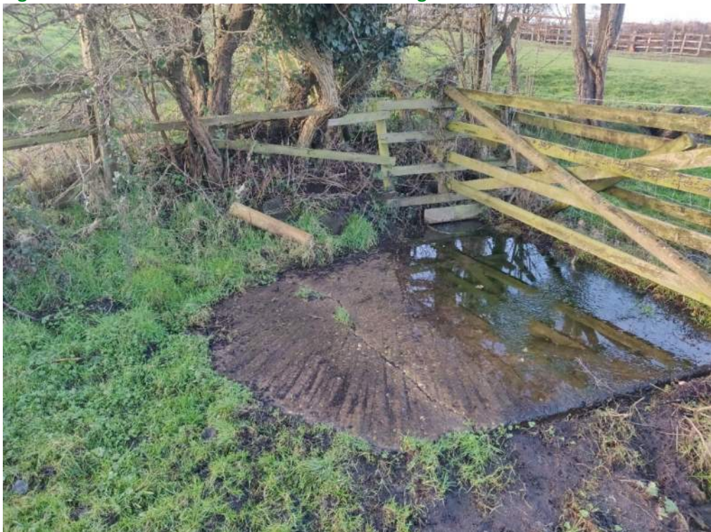
Figure 2.3: OS Marked "Pond" Area with standing water – 6 th December 2024
