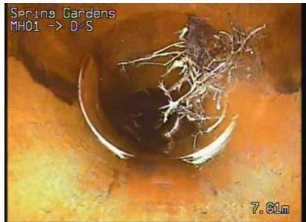
5_MH01_Downstream_DS.jpg, 00:01:41, 7.61 m Roots, mass at joint, 10% cross-sectional area loss
