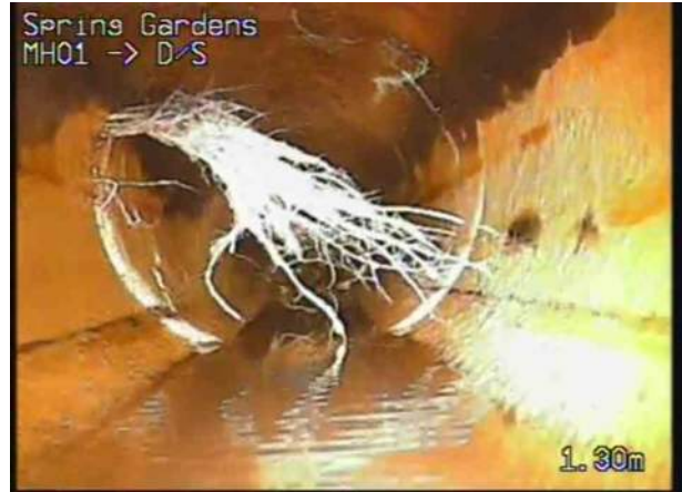
3_MH01_Downstream_DS.jpg, 00:00:41, 1.30 m Roots, mass at joint, 10% cross-sectional area loss
