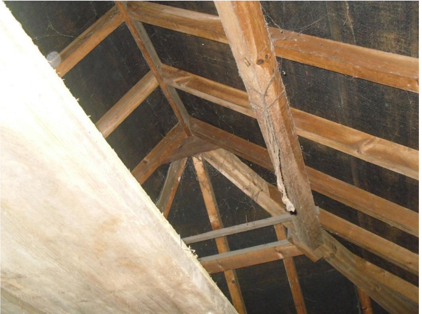
Roof interior (garage): cobwebbed
