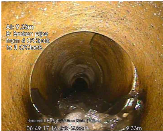
5, 00:01:04, 9.33 m Broken pipe from 4 o'clock to 8 o'clock
