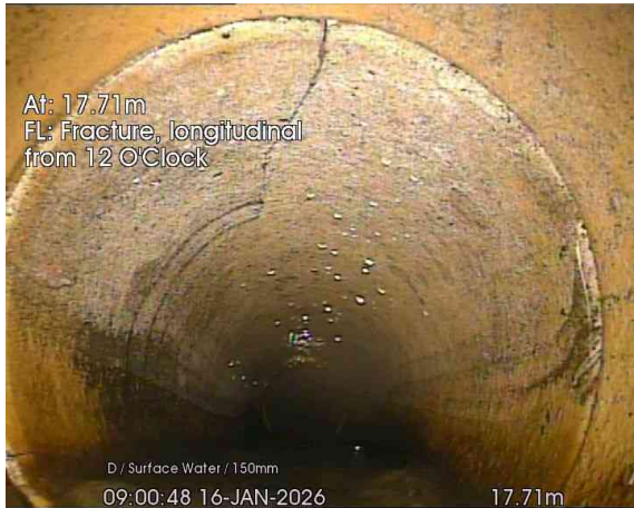
5, 00:02:05, 17.71 m Fracture, longitudinal at 12 o'clock
