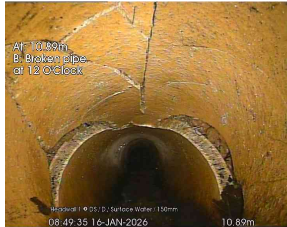
6, 00:01:17, 10.89 m Broken pipe at 12 o'clock
