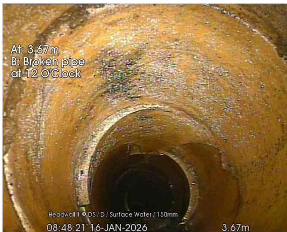
3, 00:00:34, 3.67 m Broken pipe at 12 o'clock
