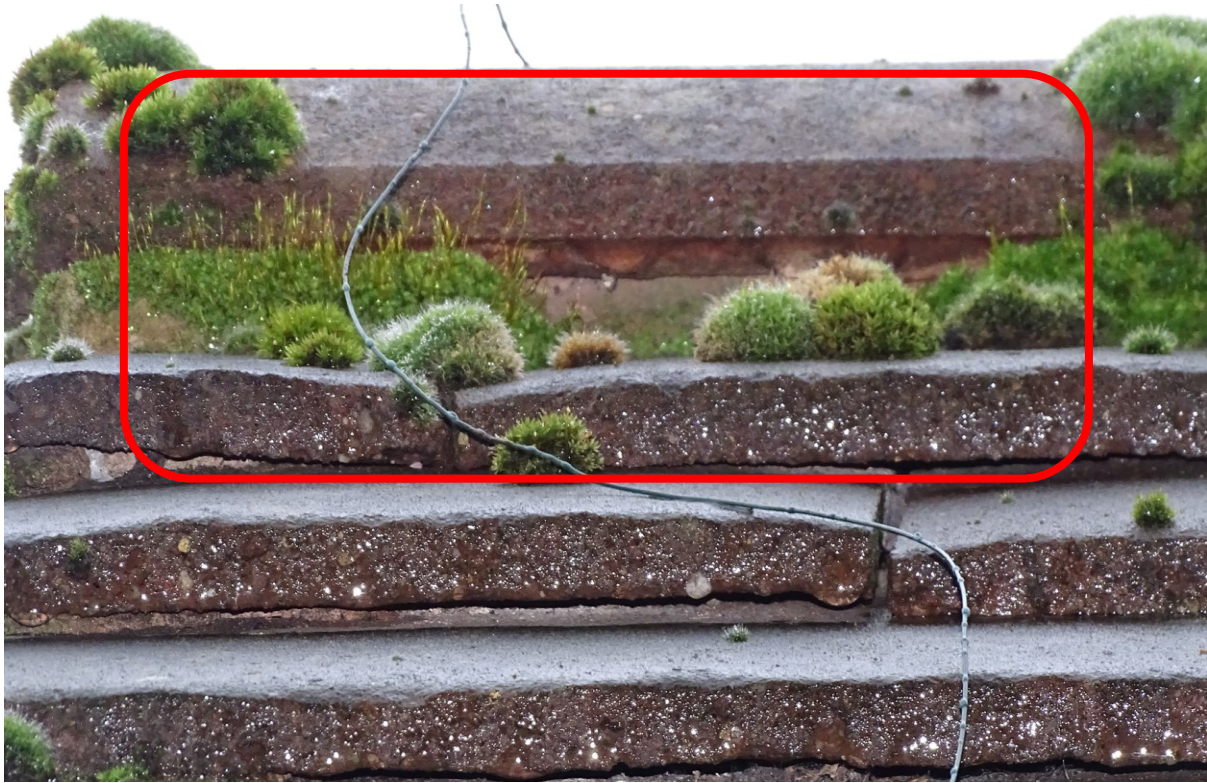
Image 9 – Gap below the ridge areas of the detached outbuilding which looks to offer adequate access opportunities for bats
