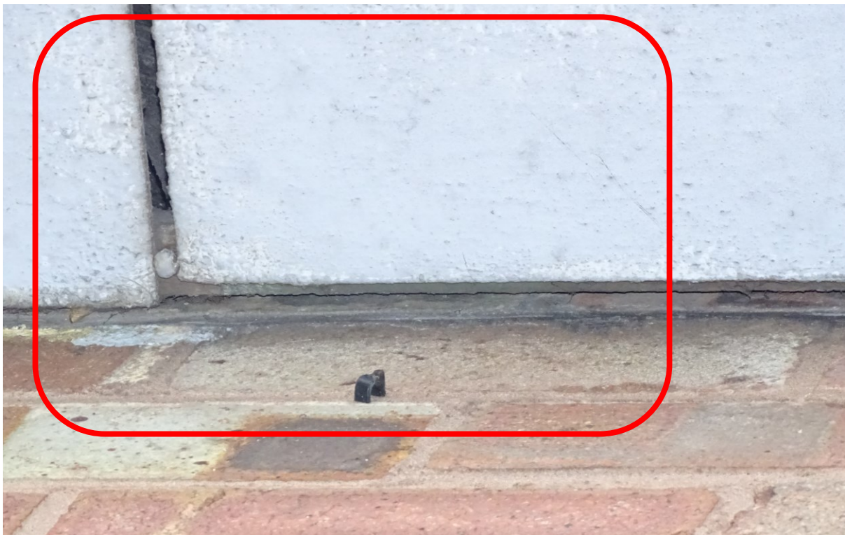
Image 4 – Gaps of adequate proportions to offer access opportunities for bats within the rear eaves coverings of the property
