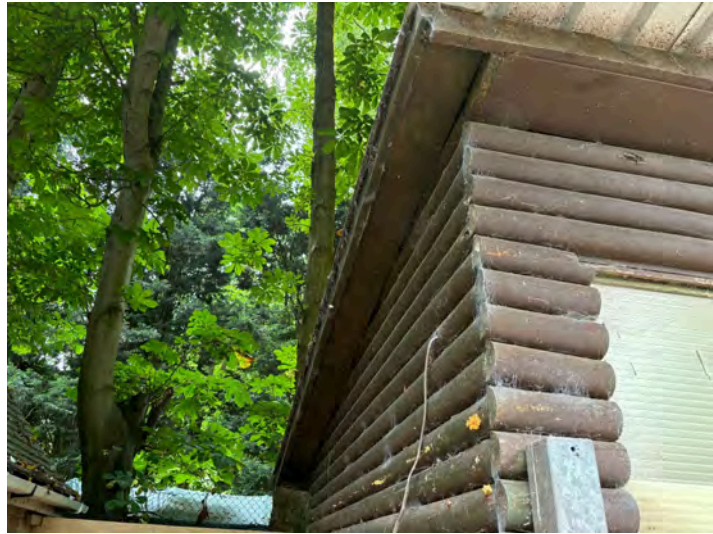
Image 10 - Condition of soffits and fascias of B2.
